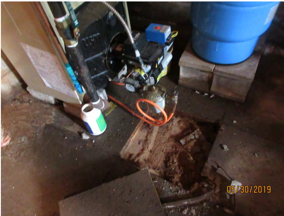
View of oil burner in basement of number seven. Floor tile removed to collect soil sample.
