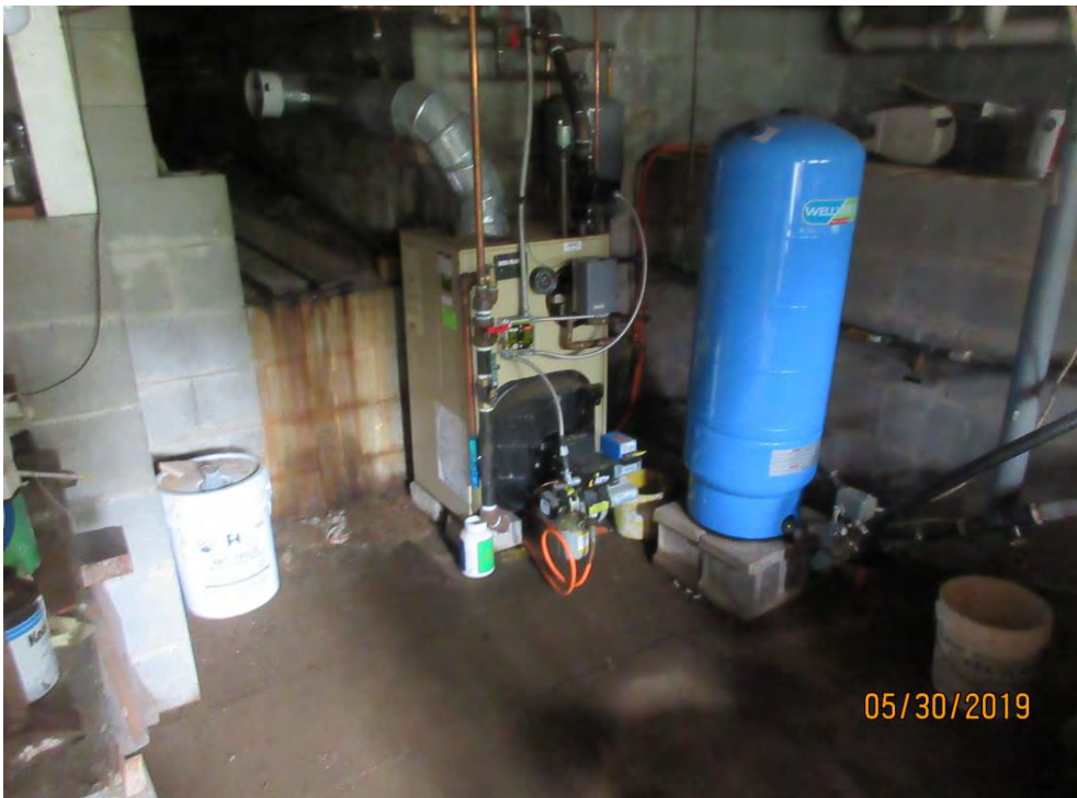
Stained floor in # 7 basement
