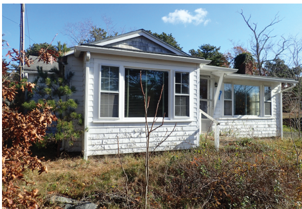
Non-compliant entry stairs at front and paint degradation.
