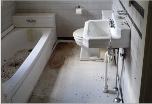
View of bathroom with non-compliant sink fixture, a bathtub with non-compliant hardware, and an outdated toilet that needs replacing.
