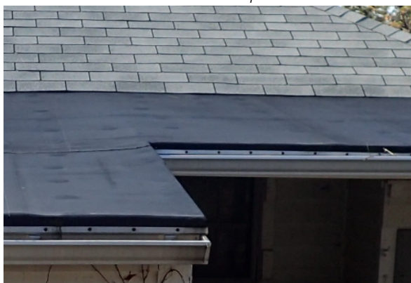
View of membrane roof of the rear addition, this roof has a significantly lower pitch than the original roof, and is showing signs of deflection in the structure.
