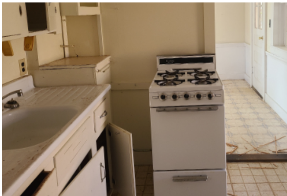
Stove/oven unit is outdated and needs replacing. There is no exhaust fan above the propane gas fueled burners.
