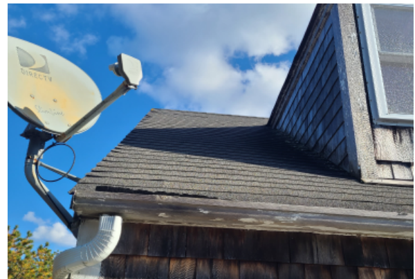
Rotted Integral wood rain gutter and downspout are rusting and failing.
