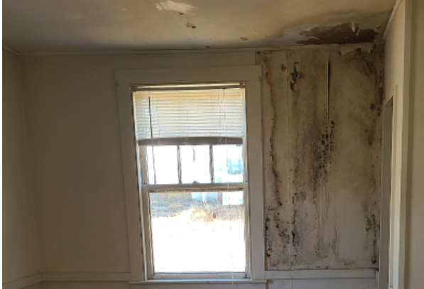
Interior wall with severe water infiltration and resultant mold.
