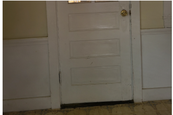
Door threshold in relation to the floor deflection, indicating a sloping settling foundation.
