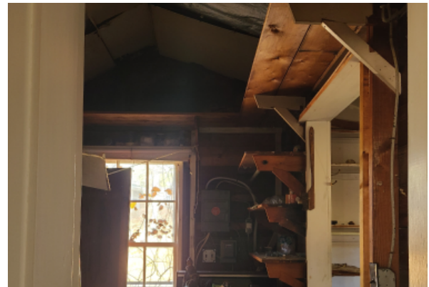
View into side addition, walls lack interior finishes revealing open stud bays without insulation.
