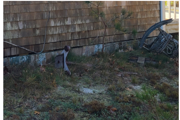
Rotting wooden foundation enclosure at grade.
