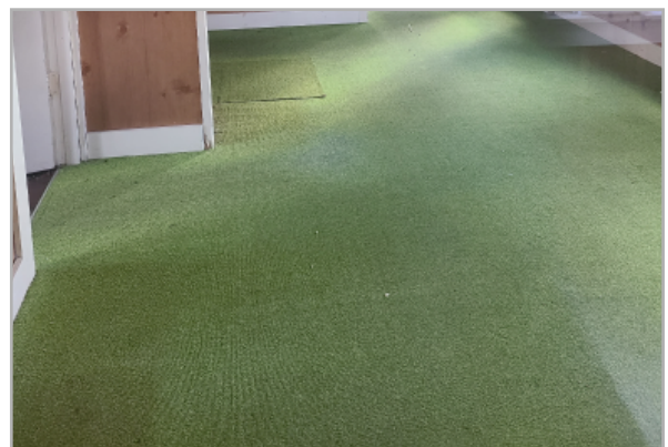
Synthetic grass carpeting covers a severely uneven wood floor surface due to sagging, undersized floor joists and foundation settlement. .
