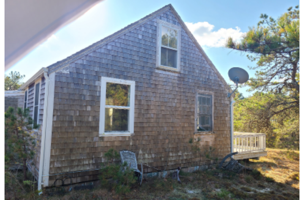
North elevation shows staining indicating water damage at each window sill.
