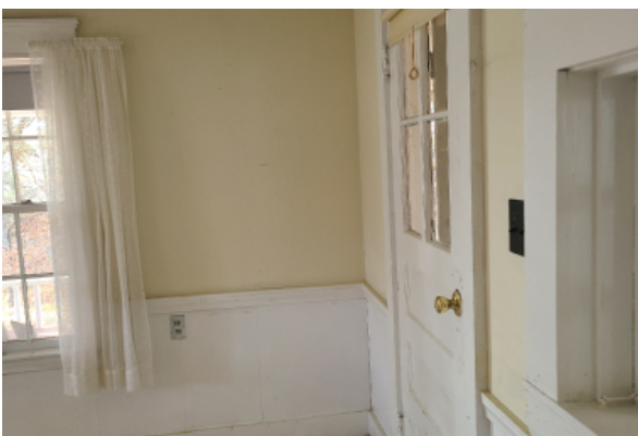
Painted plaster wall with cracks occurring due settling foundation and undersized floor joists.
