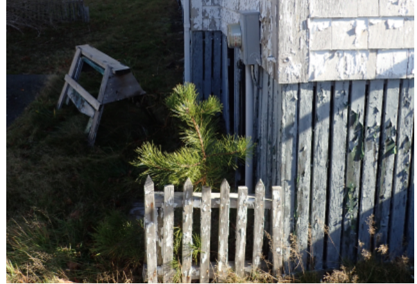
View of the foundation enclosure at the front of the building where the grade is the lowest. The boards of the enclosure are rotting and two layers of paint can be seen peeling.
