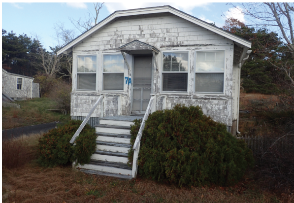
Front of cottage, front canopy roof assembly are rotted and insufficiently supported. Fascia board can be seen to be rotting as well.
