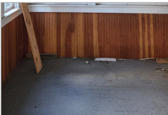
Painted sloped wood flooring at front entrance porch with stained bead board cedar wall panels.
