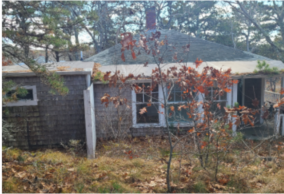
Northern face of the buildin. Most windows are single paned wood windows lacking aluminum storms. A few windows have wood framed storms.
