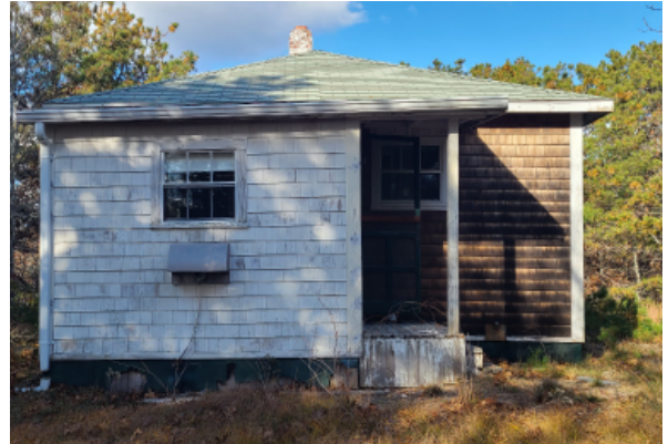
Rear elevation of kitchen addition accessed by decaying wood stairs.
