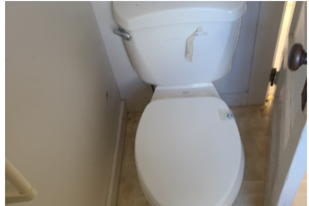
Toilet fixture in non compliant location.
