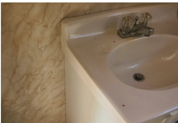
Bathroom fixture with non-compliant hardware.
