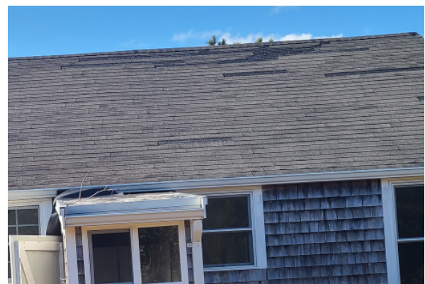
Asphalt roof generally is failing, and the shower stall addition has failed at the connection to the main structure.
