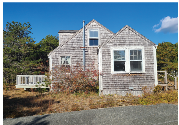
Unpainted cedar shingle siding in fair to poor conditions dependent upon wall orientation.
