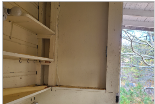
Kitchen addition wall has an unfinished interior with chipping and peeling paint. Due to the age of the structure, lead paint is assumed at all painted surfaces.
