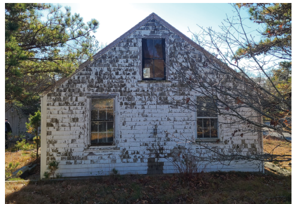
North elevation, cladding shows mold growth and paint has peeled from almost 50% of this face.
