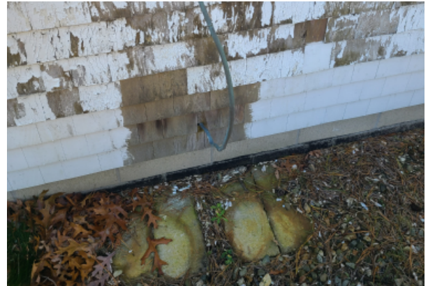
CMU perimeter foundation with grade build up, and insufficient water mitigation.
