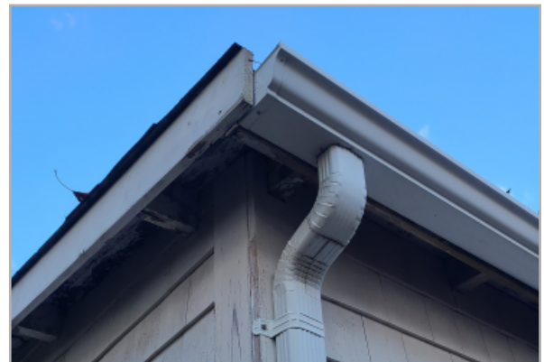
Rake trim at asphalt shingle termination is failing.
