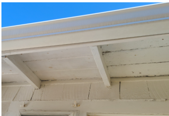
View of the roof eave condition where the paint is chipping between the sheathing boards. The peeling is not uniform throughout indicating that the roof eave may only have water penetration in just those areas.
