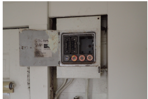
Conduit box with original fuses is non compliant and must be removed and replaced with up-to-date fixture and wiring.
