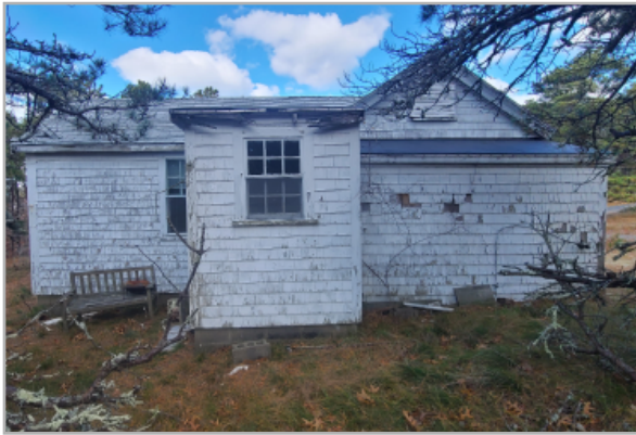
South face of the building, the paint is peeling and chipping on almost 80% of the wall surface area.
