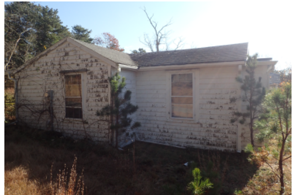
North face of building where exterior walls meets grade. Peeling and chipping of paint from the bottom up indicated water penetration from the base of wall.
