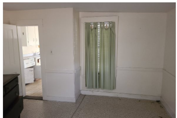
Painted plaster wall with signs of mold and mildew growth. The window in this room is now interior due to the side addition.
