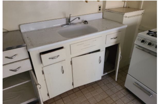
In counter sink and cabinet storage underneath. The cabinets and drawers could not close due to warping and the deflection of the floor structure below.
