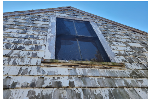
North side peeling paint and rotted window sill. Window lacks storm.
