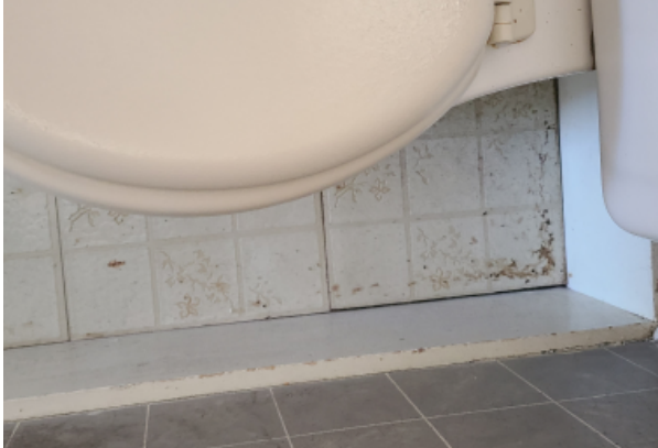
Sheet tile flooring in full bathroom. Tiles have become unsecured in areas and failing.
