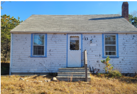
Asphalt shingle roof showing nonconformities and failure of adhesion in places.
