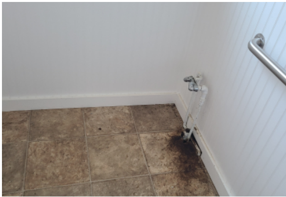
Missing bathtub fixture.
