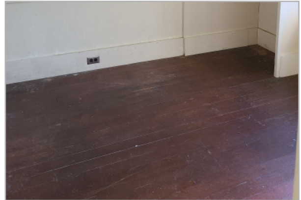
Wood flooring in bedroom is in fair condition. Non-grounded electrical outley located in baseboard.
