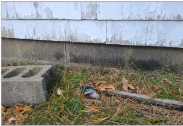
CMU foundation with discoloration indicating water damage within, and cracking in the mortar joints.
