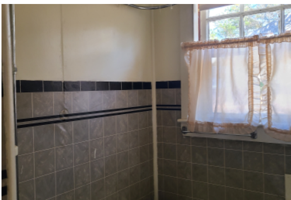
Tile wall finish in full bathroom, terminating in a tile bull nose and has painted plaster above.
