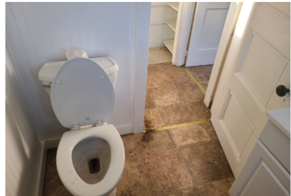
Toilet fixture and sink, the layout of this bathroom is non-compliant with accessibility codes.
