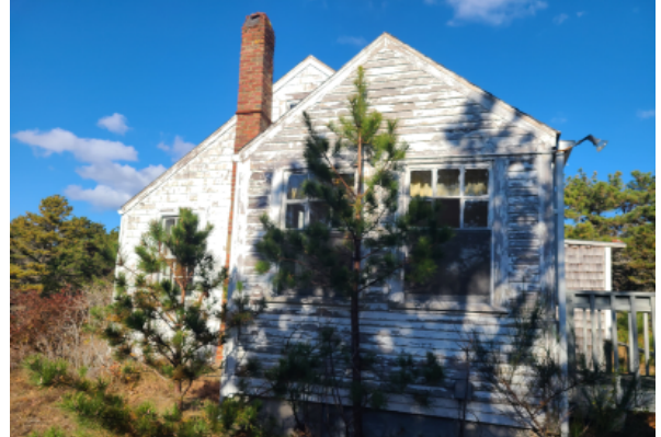
Southern face of the building kitchen addition with newer windows than the rest, but still insufficient due to age.
