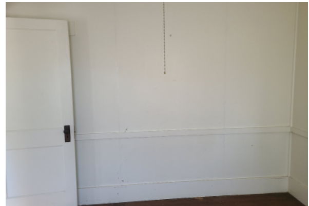
Painted plaster wall with corner and base trim, with trim board at about 3' above finish floor. Paint shows signs of mold growth and the seams between panels have become visually apparent.
