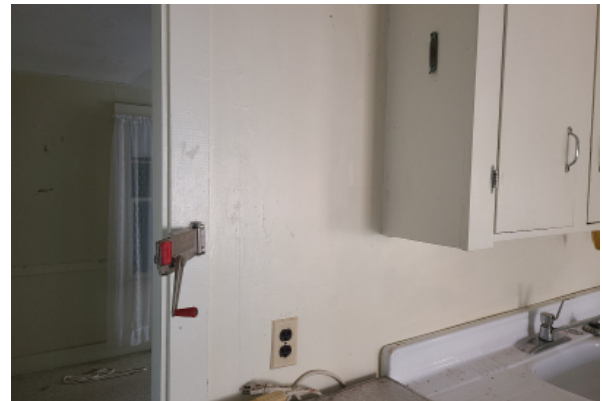
View of kitchen wall with dangerous non-GFCI, non-grounded electrical outlet next to kitchen sink.
