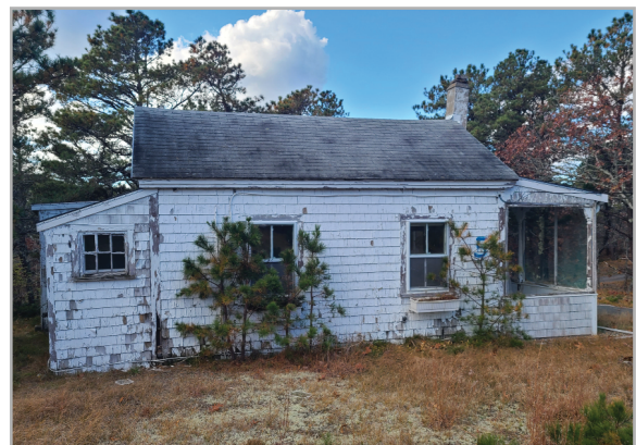
Building siding paint is peeling throughout with rotting deteriorated shingles and wood trim boards.
