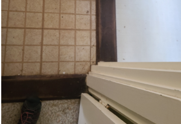
Condition of floor finish transition. Floor plan at this location is not wheelchair accessible due to configuration of cabinets and doorways and door thresholds.
