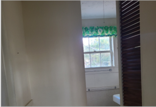
White plaster walls in bathroom is showing signs of mold and mildew growth.
