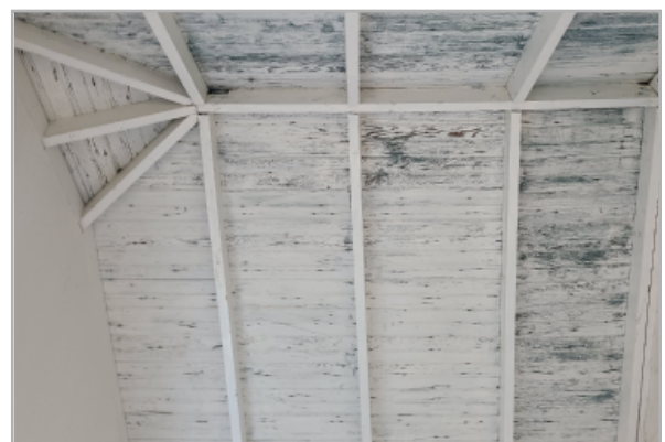
Interior of roof in front porch addition, with peeling paint and signs of water ingress.
