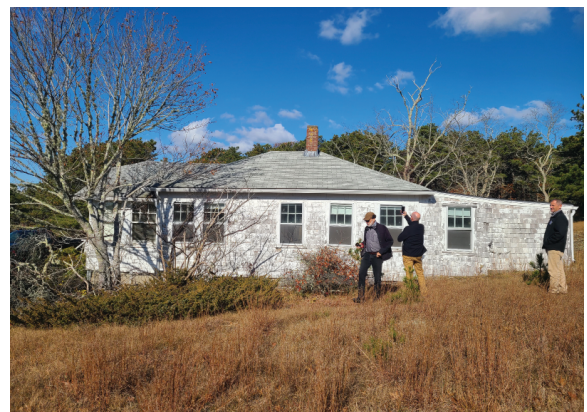
Southern face of cottage, front and rear additions are apparent. This face is missing at least 50% of its paint.
