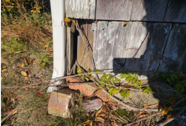
View of foundation pier, wood siding, wood foundation skirt, and brick supports. Foundation is insufficient for this building, and was not intended to support two levels.
