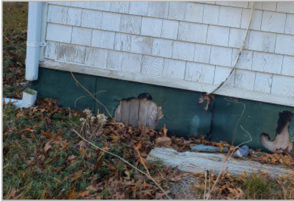
The foundation skirt has rotted through a damaged membrane layer.
