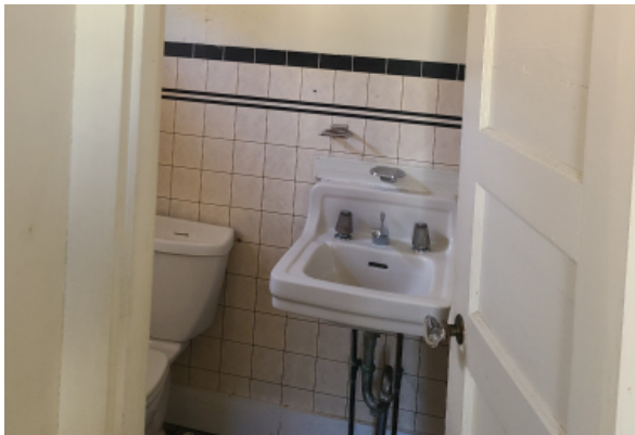
Half bath with sink and toilet. Sink fixture is non compliant.
