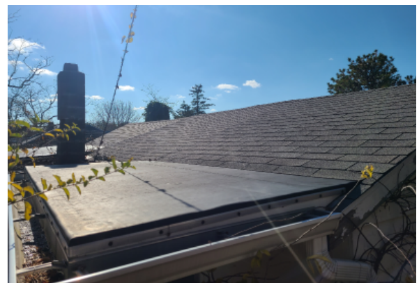
Membrane roof condition of building additions with signs of degradation.
