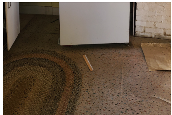
Sheet flooring that is badly worn with visibly evident floor deflection throughout.
