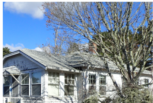
Cottage roof condition with front addition roof rake meeting the original building siding below the original roof eave. This roof construction is non-compliant and must be made to be so.
