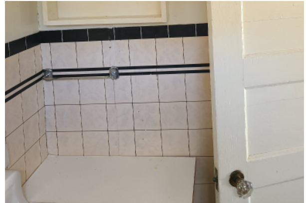
Tile wall finish in half bathroom, terminating in a tile bull nose and has painted plaster above.
