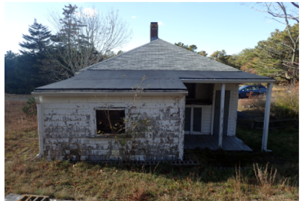
View of rear addition to the East, the paint has chipped and peeled off of most of the siding. The window in this wall shows signs of water penetration about the perimeter.
