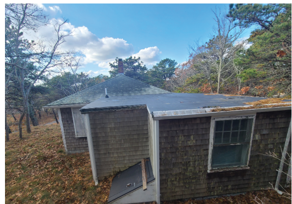
View of East elevation, there is a rear addition, with discoloration throughout siding indicating water damage.
