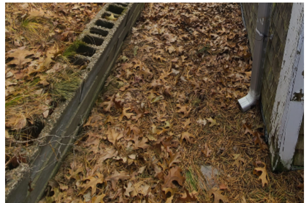
CMU retaining wall off set from foundation does not provide enough depth to keep the exterior building envelope from contacting the ground resulting in rotting and decaying of the exterior wall fabric in this location.
