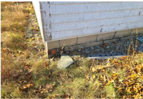
CMU foundation wall at grade, with brick patching seen in the corner.
