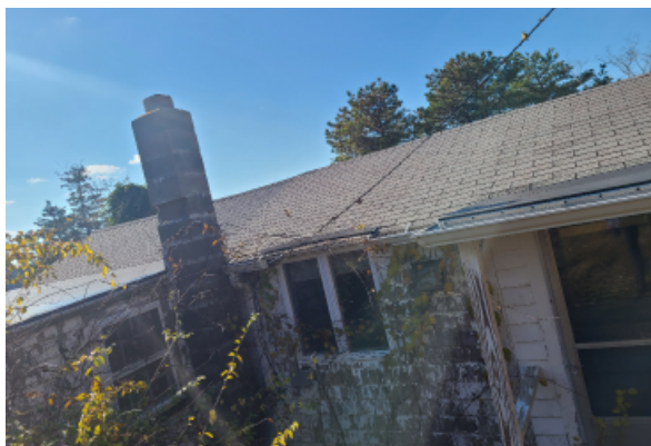
General roof condition, the shingles show little sign of deflection but their adhesion and viability are assumed to be insufficient due to age.
