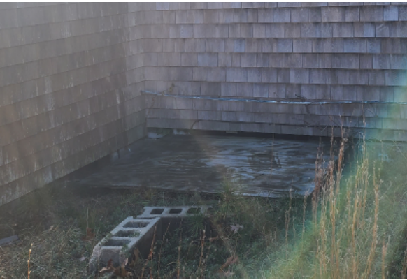
Rotting wooden access hatch to foundation crawl space, and remnants of CMU retaining wall.
