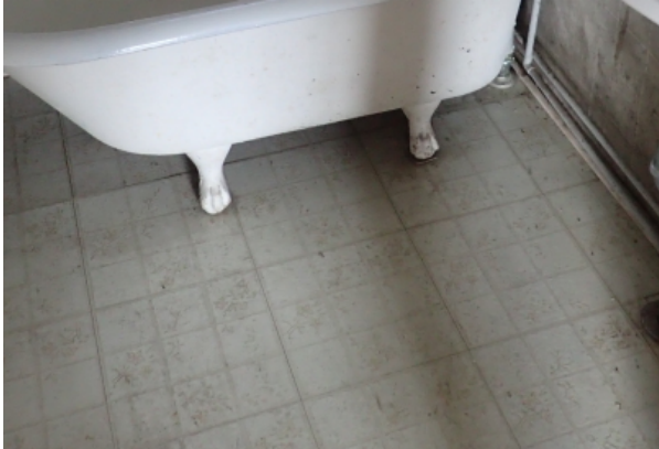
Sheet tiling in bathroom that is crumbling at the edges and seams.
