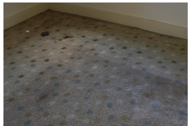
Sheet flooring in bedroom, evidence of water damage, and is crumbling at the edges due to age.
