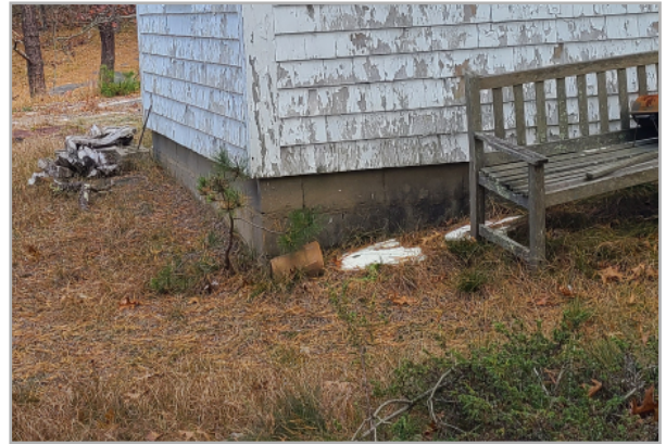
View of CMU foundation at South West corner, vegetation is beginning to encroach and the presence of a tree sapling suggests root penetration.
