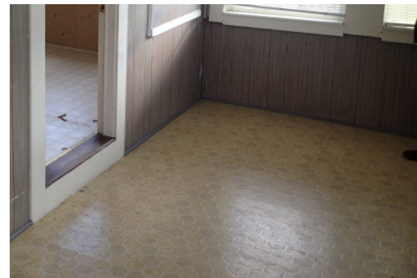
Change in material between rooms, and significant change in floor elevation. Floor sheet finish shows signs of deflections throughout.
