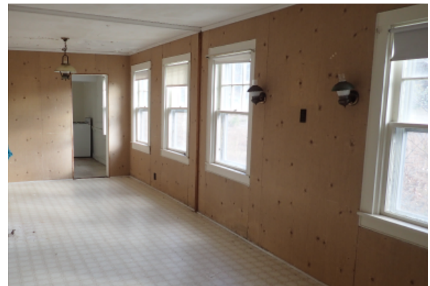
Floor to ceiling wood paneling with base and crown molting. There is some rippling indicating some deflection occurring from the interior structure.
