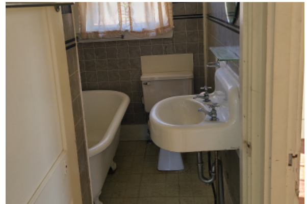
Full bath with toilet, sink, and bathtub. Sink fixture is non compliant, and bathroom layout is unacceptable by code.
