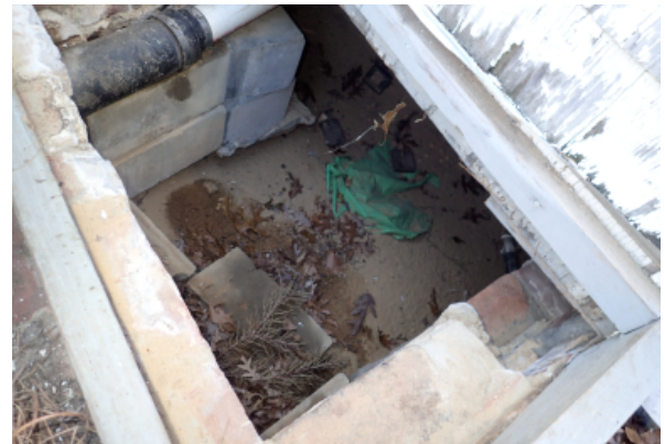
Access to foundation crawl space, the foundation of CMU and wood members can be seen.
