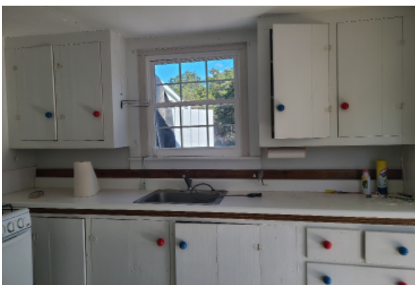
In counter sink, with missing and non compliant hardware. Cabinet hardware is also non compliant.
