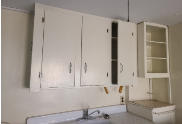
View of kitchen cabinetry and in counter sink. The hardware for the sink is non-compliant, and the cabinetry needs replacing due to structural concerns.
