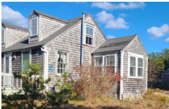
Asphalt roof above kitchen addition shows insufficient roofing coverage.
