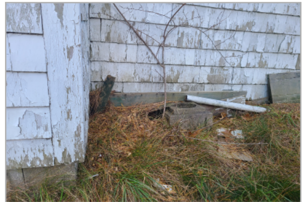
Ground and debris built up against CMU foundation and wall cladding at Southern elevation. Voids in the wall allow animals to enter and live under the building.
