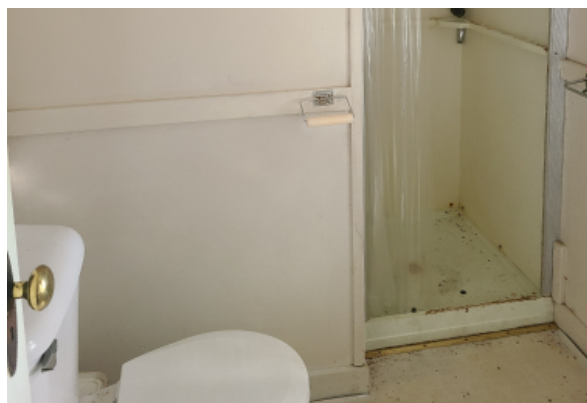
This building has a toilet, sink, and shower stall. The shower stall needs replacement due to degradation of materials.
