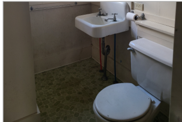
Wall hung sink with separate hot and cold faucet fixtures. Hazardous non-GFCI, non-grounded electrical outlet next to sink.
