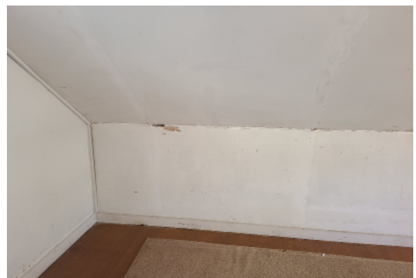
Variable wall heights at second level with trim board at borders, paint is chipping and peeling throughout.
