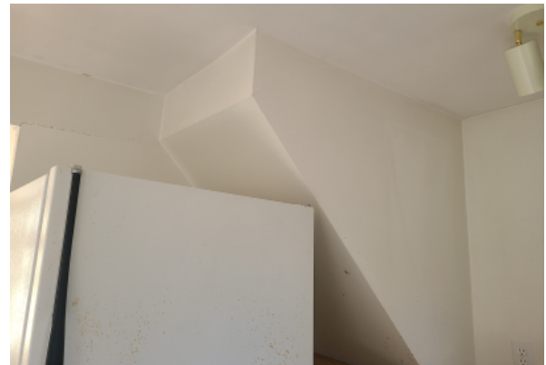
Sloped ceiling condition below stairs, enclosed with plaster and painted to match.
