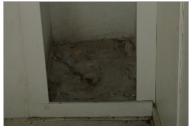
Bathroom flooring is sheet tile, and has areas of mold growth and discoloration. The floor of the shower stall and base of wall is covered with mold and mildew growth.
