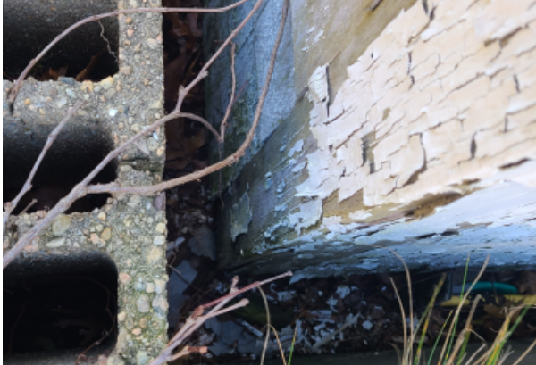
View of CMU retaining wall slightly offset from building siding. Paint has peeled from the base of wall up, indicating water has penetrated the CMU to the siding.
