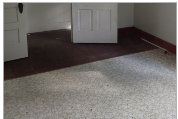
View of room floor with two types of flooring and flush doorway threshold. The flooring is chipping and damaged in areas and must be replaced.
