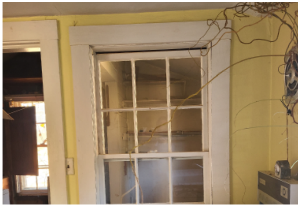
Exterior window that became interior with the side addition. To the right is a through-wall exhaust fan with vegetation penetration.
