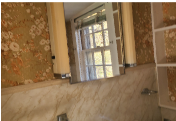
Wallpaper and marble wall finish in bathroom. The wallpaper is showing signs of mold and mildew.
