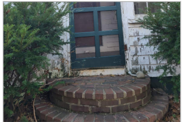
Brick steps at front entry. Note rotting shingles at bottom courses to brick.
