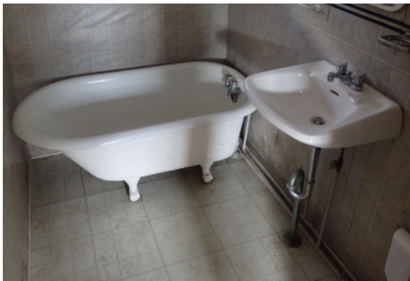
Sink and bathtub, both with non compliant hardware. Toilet is also present as well in this bathroom.
