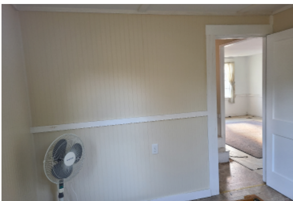
Painted plaster wall with trim at base, mid, top, and about doorways. Paint is yellowing due to age.
