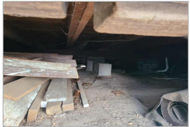
View to crawl space showing notched 2x6 beams and 2x6 wood floor joists. The exposed underside of this and many of the other cottages creates a potential habitat for wildlife.
