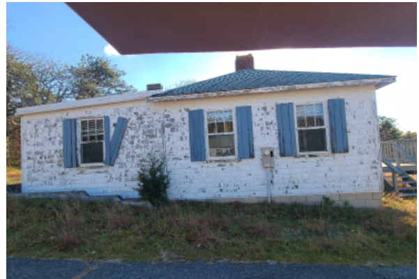
North elevation, bedroom addition to the left has with damaged window and peeling paint.
