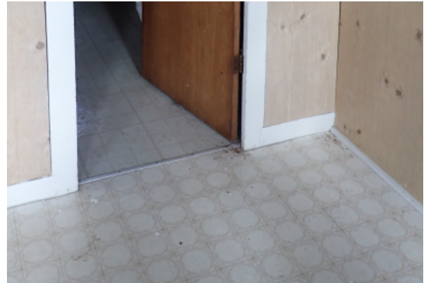
Sheet flooring with signs of degradation throughout and crumbling at the edges.
