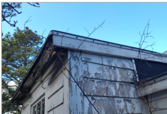
View of back additions, the membrane roof has failed and the fascia board has rotted out exposing the structure behind to the weather. The building siding has also been patched with a membrane sheet to the right.
