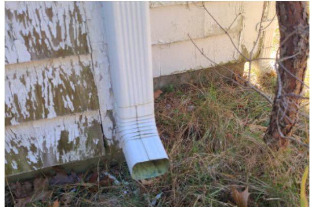
View of the base condition of a downspout where the last length of aluminum is missing. The water run off is insufficiently removed from the building footprint.
