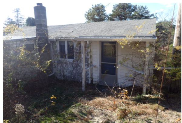
Rear elevation of the building where vegetation has penetrated the exterior chimney and into the building interior at open penetrations. Roof edge areas unprotected by a gutter lack paint and shows signs of decay.
