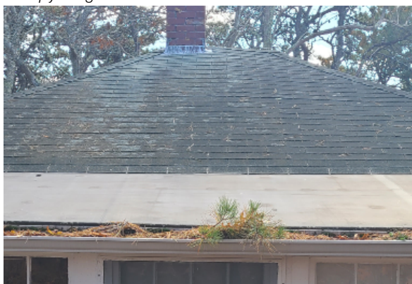
View of side addition membrane roof in relation to the original hip roof. The asphalt shingles are beyond their useful life. The gutter is filled with organic material supporting vegetative growth.
