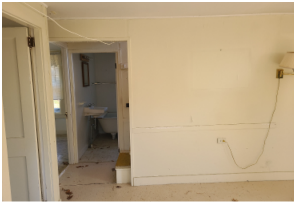
Painted plaster walls with crown molding. Paint is yellowing and peeling.
