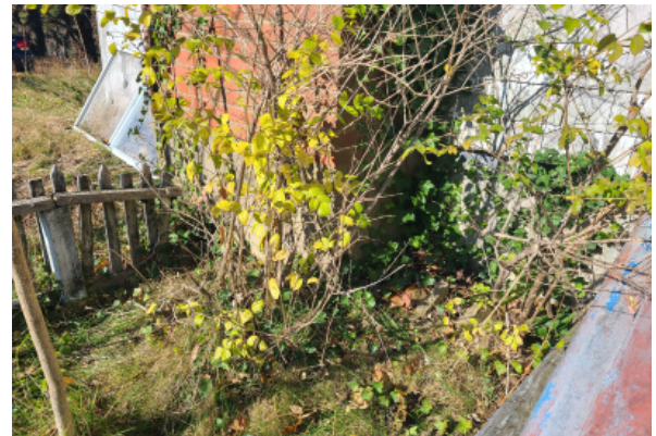
View of vegetation overgrowth penetrating chimney and wood shingle siding.
