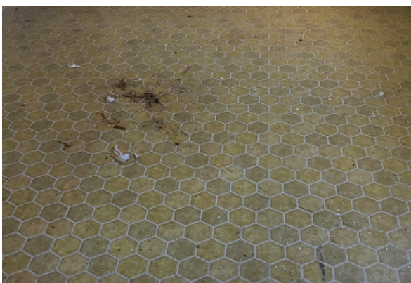
Worn and damaged sheet flooring.
