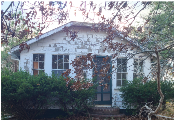
Front addition. Brick mortar steps, and peeling paint on shingle siding and fascia, rake, door and window trim
