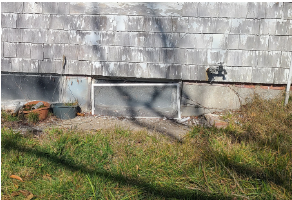
View of cracked parged CMU foundation. The basement window in this area is missing, allowing for animal habitation.
