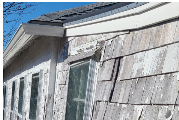
View of the original asphalt roof construction connecting to the rear addition membrane roof rake. The ridge of the original roof can be seen to show signs of degradation.
