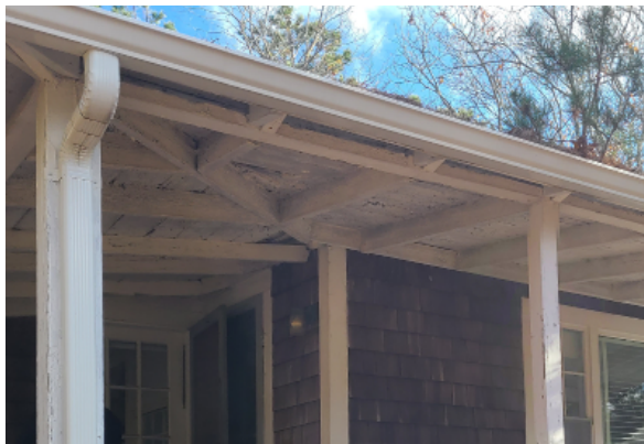
Front porch addition roof is an extension of the original roof and is secured into the exterior wall structure. The building structure is insufficient to support the porch canopy weight
