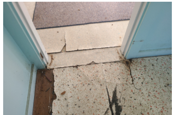
Piece made sheet flooring crumbling at the edges. Multiple layers of flooring can be observed in the area at the top of this photo. The area at the bottom has large areas where the flooring has crumbled to reveal the floor sheathing.
