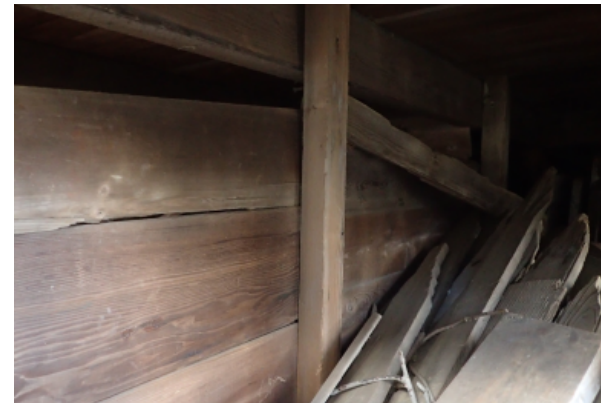
View into foundation crawl space. Insufficient floor supports can be seen, and a wood board partition dividing the space into storage and inaccessible.
