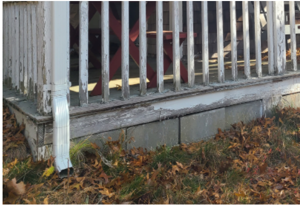
CMU on grade foundation for porch addition is an insufficient structure, and the wood framing is in contact with the ground on the northern side (left).
