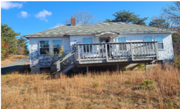
Shingled eyebrow canopy over front entry is rotted and failing. The fascia board is damaged and rotting at the entire perimeter of the roof. The wood deck is not worth saving.
