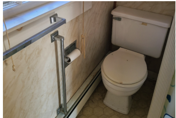
Toilet fixture with signs of damage due to normal wear and tear. There are nonconforming guardrails in this location as well.
