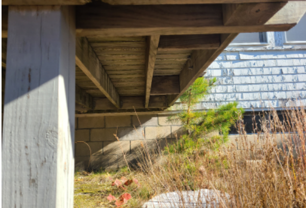
Deck addition framing supported by the CMU foundation at one side and piers at the other.
