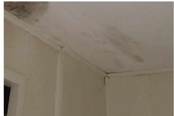
View from the interior of water damage and mold seen in the ceiling indicating multiple areas of water penetration into the roof.
