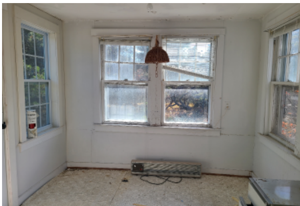
Kitchen addition, paint is chipping and peeling throughout and water damage can be seen at the windows.
