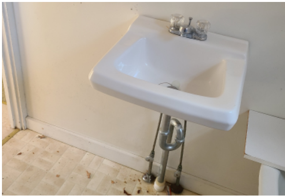
Sink fixture with non compliant hardware and uninsulated non-compliant piping below.
