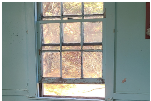
This window stuck open, exposing the interior to the elements.
