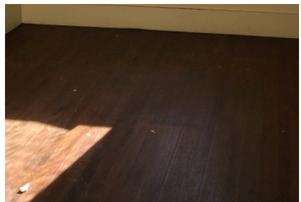
Hardwood flooring needs restoring, and has a slight pitch indicating foundation settlement.
