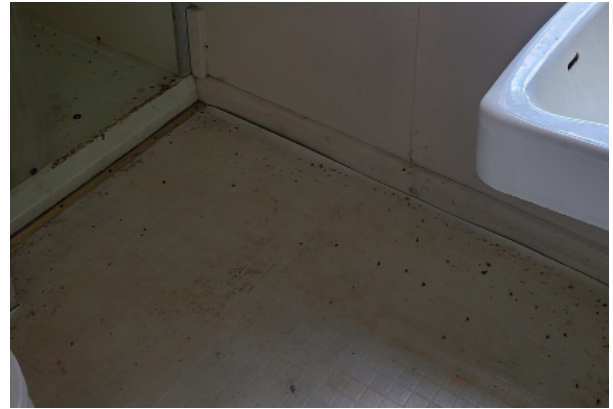
Sheet flooring in bathroom with signs of degradation throughout and crumbling at the edges. Signs of water damage are apparent at the edge of shower stall.
