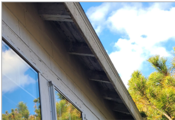
Exposed roof rafters at eave show signs of rot, and peeling paint on fascia board.
