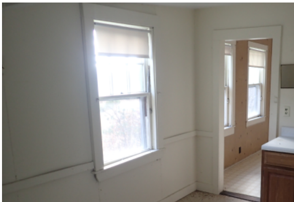
Painted plaster wall with trim about openings and at the base, as well as trim board at about 3' above finish floor. Paint shows signs of mold and mildew growth.
