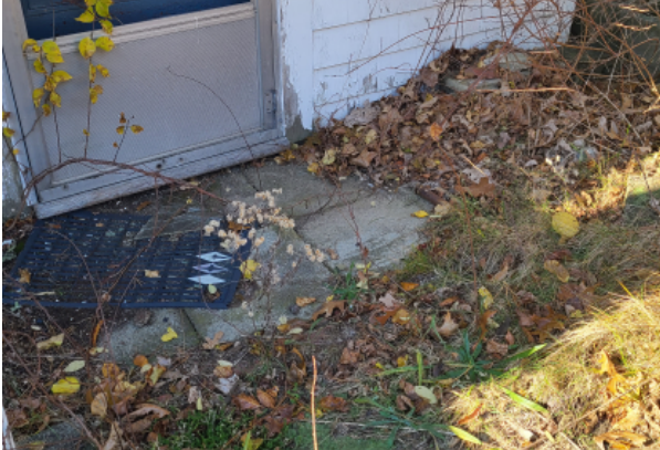
Concrete landscaping tiles at grade at the back entry to the building that have become obscured by the ground and vegetation encroachment and must be rehabilitated.
