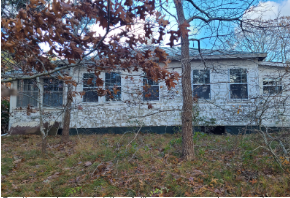
Peeling paint, and siding failing at penetration openings and rotting at the roof line. Additions to the left and right.
