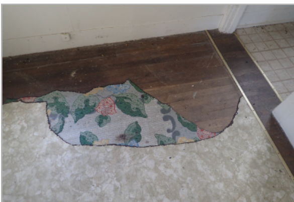
View of multiple layers of floor coverings that have crumbled away to expose the original wood floor blow. Sagging and sloping of floors and evident wall cracking suggest the foundation has settled over time.
