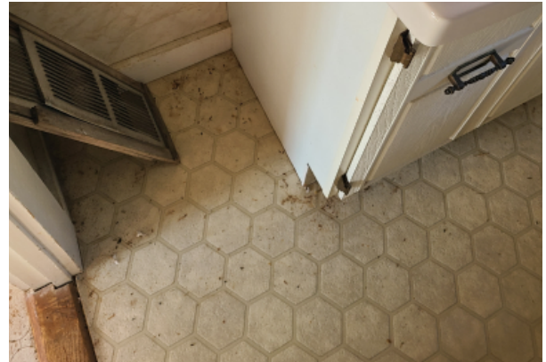
Sheet flooring that is degrading and crumbling at the edges.
