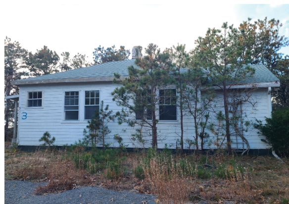
Side elevation with missing rain gutters and overgrown foundation plantings
