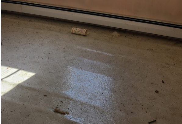
View of sheet flooring with evident signs of deflection occurring.
