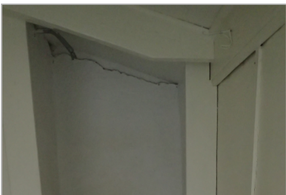
View of crumbling wall and ceiling due to insufficient moisture protection, and must be investigated for extent of damage.
