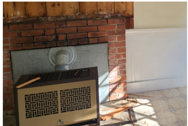
Propane fueled central heating unit with signs of water damage from the chimney.
