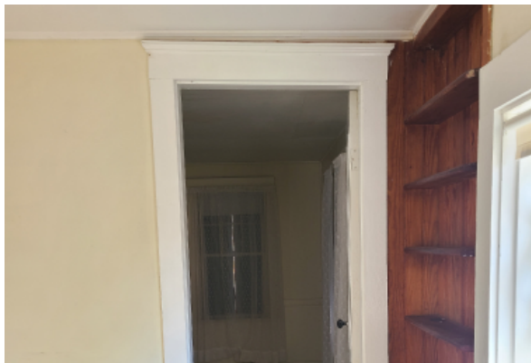
Interior door frame that is tilted, illustrating the failing foundation. This entire front room is sloping out from the central point of the inner most wall (facing here). The door opening width is 26\"/>
