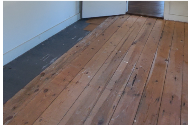
Buckled wood flooring in one of the bedrooms due to water damage.
