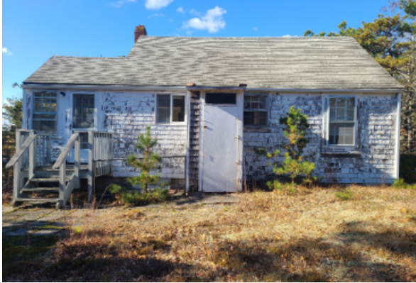
View showing wooden steps into kitchen addition that are rotting due to age, and an exterior accessed shower stall attached to the back of the building.
