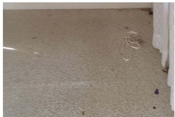
Sheet flooring with signs of degradation throughout.
