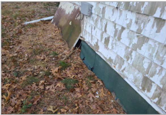
Deteriorated painted plywood foundation skirting.
