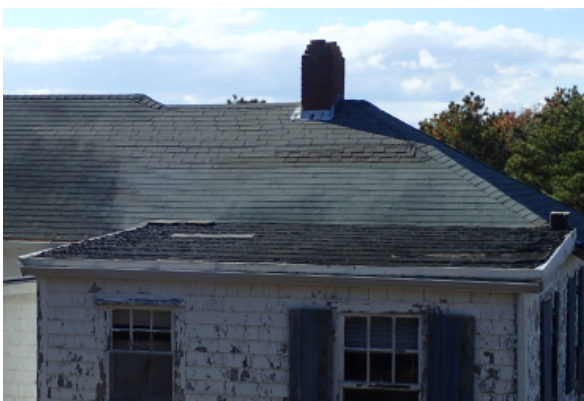
Poorly constructed addition with degraded asphalt shingled low pitched shed roof.
