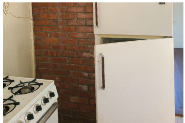
Oven/stove fixture and refrigerator. Both require replacing due to age.
