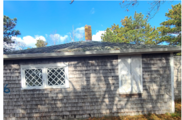
Southern face of the building, with one window opening boarded up. The sill of the covered window is rotted with signs that it is allowing water into the building.
