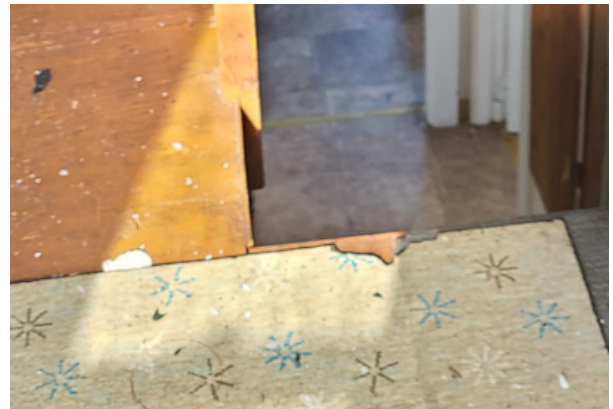
Sheet flooring and board flooring at second level, crumbling and failing from age.
