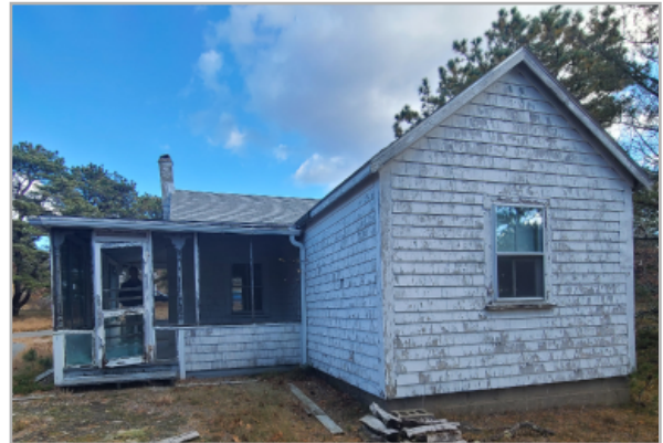
View of West face of building, the paint is peeling and chipping off of almost 90% of the surface area. The front porch addition is failing as is the masonry chimney.
