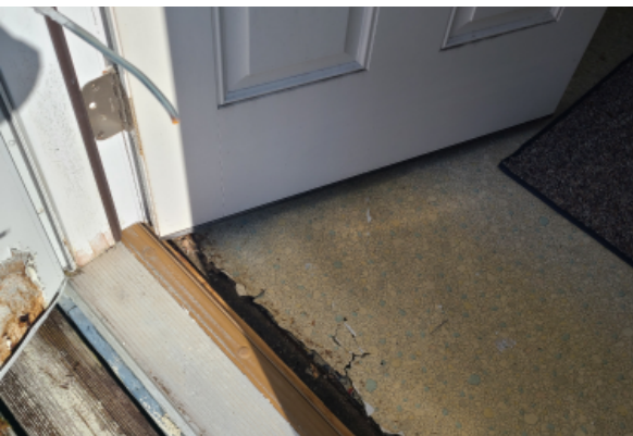
Sheet flooring at building threshold is damaged down into the floor sheathing and crumbling.
