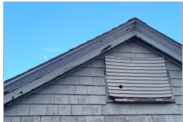
A view of the rake condition of the original roof. A louver is located at the peak, and has deflected out of its penetration. The rake shows sign of mold between the fascia board and siding.
