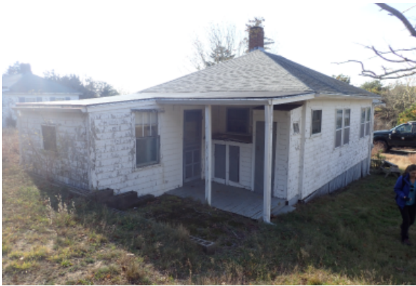
There is a covered porch at the rear of the cottage, with a shower stall and cabinets. All painted surfaces are chipping and peeling, and signs of mildew at the porch.
