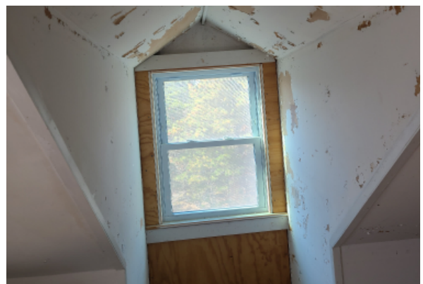
Dormer condition at the second floor. Chipping paint and insufficient framing about window.
