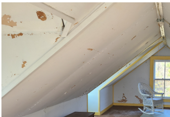
Roof from the interior of the second level. Water damage can be seen, as well as ripples indicating further damage and settling.
