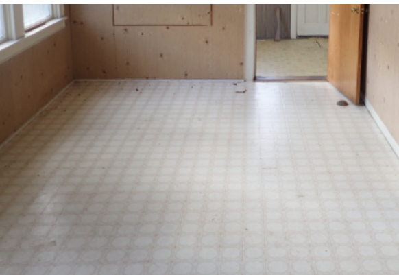
Wall to wall sheet flooring with word spots and some crumbling at the edges.
