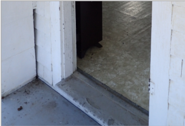
View of exterior threshold that is greater than one inch which is non-compliant with code, and deflection in the interior sheet floor finish can be observed.
