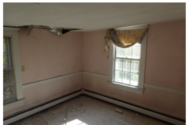
Painted plaster wall with trim about openings and at the base, as well as trim board at about 3' above finish floor. Paint shows signs of mold and mildew growth. The very low 6'-10" ceiling is open to the roof structure in one area.
