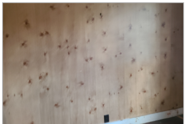
Wood panel walls, naturally stained with a contrasting base board. There are signs of mold and mildew growth in some areas.
