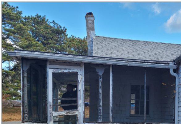
The front porch addition roof is pitched incorrectly causing water to run towards the gable end of the roof.. This entire construction has degraded and must be demolished.
