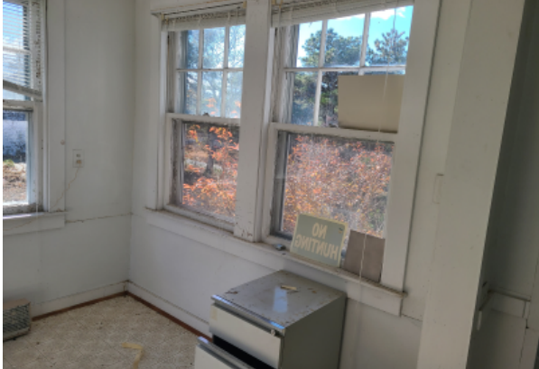
Kitchen addition windows, single paned and damaged bug netting.
