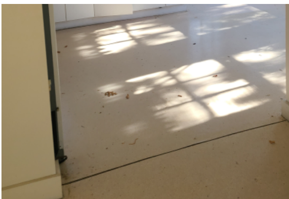
Uneven flooring transition between two rooms.
