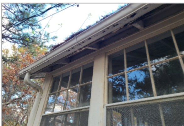
View of exposed and rotting eave with aluminum gutters sagging from the weight of accumulated organic matter supporting live vegetation.
