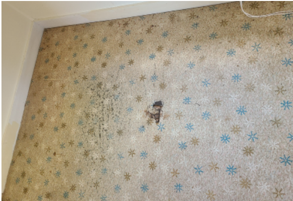
Sheet flooring, worn down to the floor sheathing in areas and crumbling at the edges.
