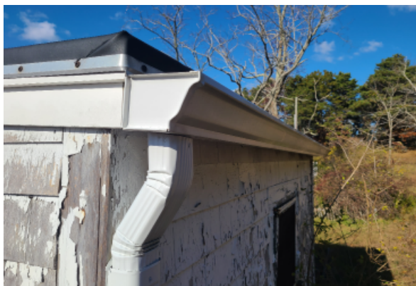
View of typical gutter and downspout condition at this cottage. The connection of the gutter to the roof eave is non-compliant, and the rust apparent in the fastening screws indicates a need for roof replacement.
