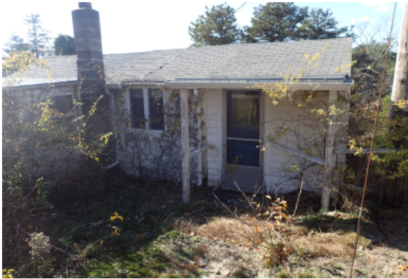
East elevation has excessive vegetation overgrowth that has penetrated the shingles in some areas.
