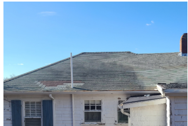
Patched asphalt shingle roof past it's useful life.
