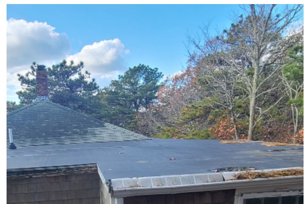
View of rear addition membrane roof in relation to original asphalt shingle roof. Evidence of ponding can be seen in the membrane roof, with vegetation build up in the gutter as well.
