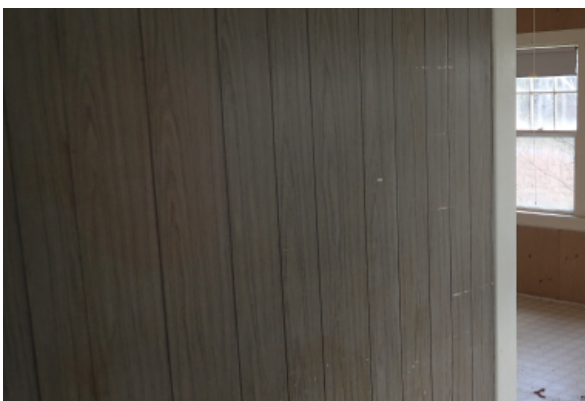
Clear wood board paneling wall finish, shows sign of mold and mildew, and there are scrapes in places as well.
