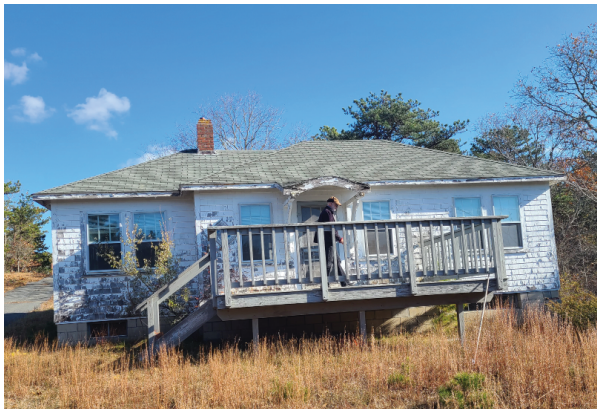
Front view of cottage, CMU foundation has two window penetrations just above grade. The paint is peeling throughout.
