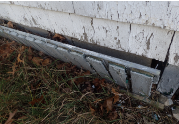
Wooden foundation enclosure rotting and detached from the building. Signs of past reinforcement efforts with a horizontal 1x3 can be seen at the very base.
