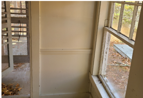
Exterior corner of side addition with painted plaster walls. The window is not protected with a storm window and is in poor condition as a result.
