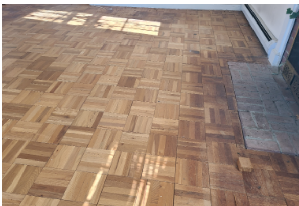
Wood parquet tile flooring with signs of warping and deflection throughout. Asbestos was detected in the flooring.
