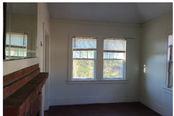
Painted plaster wall with base board trim and crown molding. Trim around window frame is beginning to separate from the wall, and needs replacing. Window hardware at the top is damaged and must be removed.
