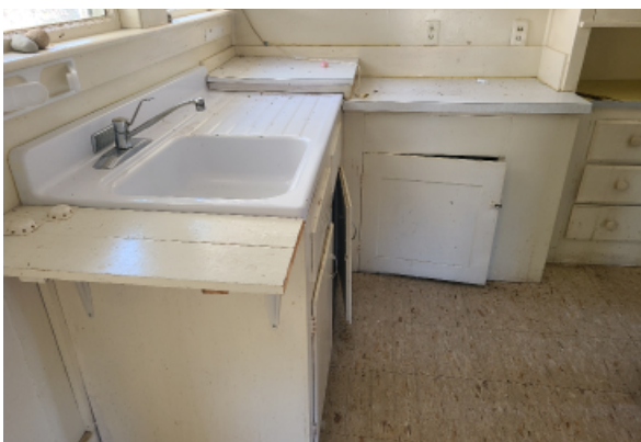
Counter sink, with non compliant hardware.
