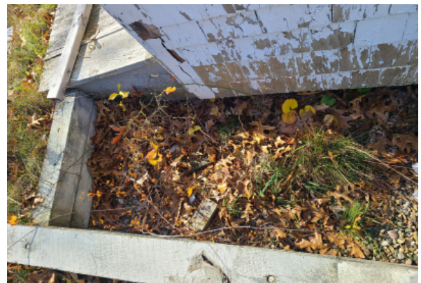
Insufficient wood retaining wall set back from building face.
