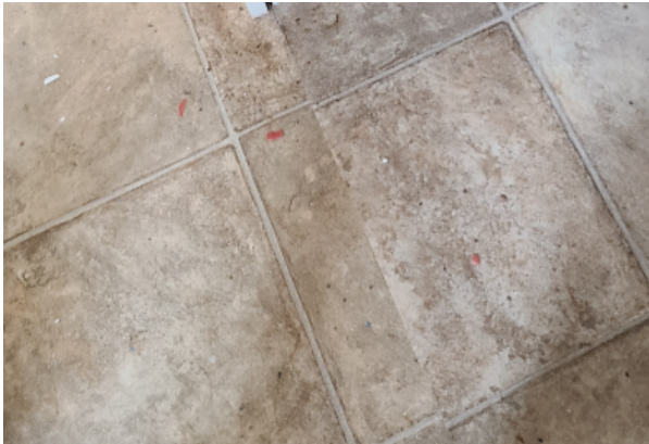
Tile flooring with failing grout joints and cracked tiles.
