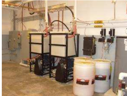
Wash Equipment Room
