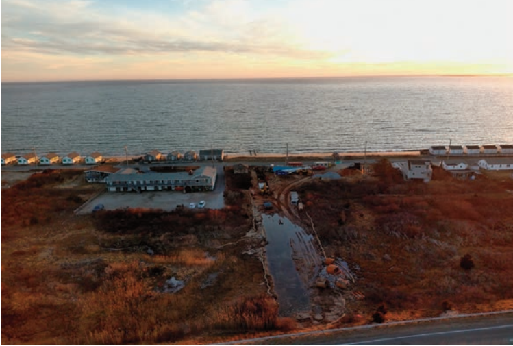
East Harbor Culvert repairs between Shore Rd and Route 6 Photo Courtesy of Jarrod Cabral
