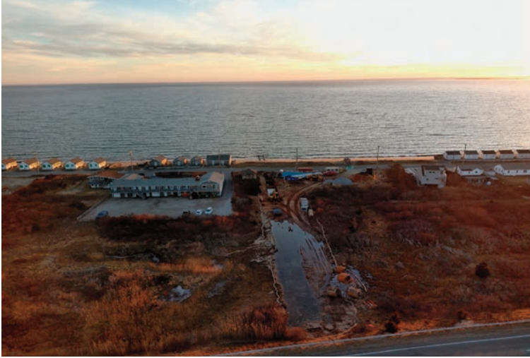
East Harbor Culvert repairs between Shore Rd and Route 6 Photo Courtesy of Jeffery Souza
