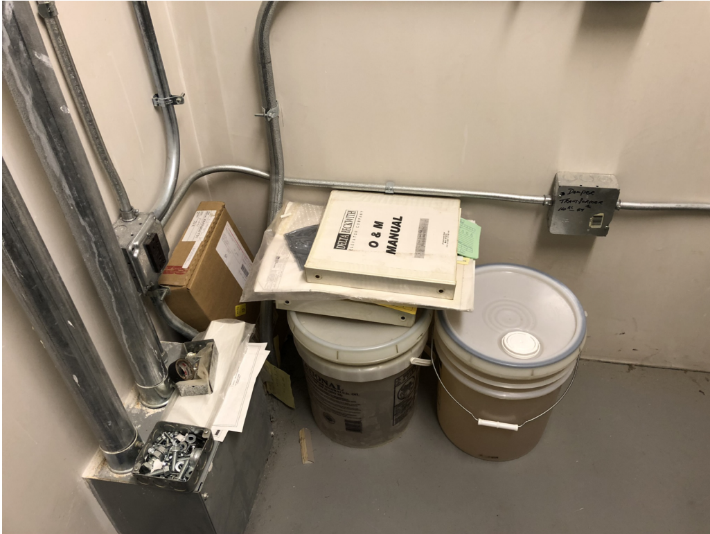
Photo 9: 5-gallon buckets of hydraulic oil adjacent to elevator pump motor.
