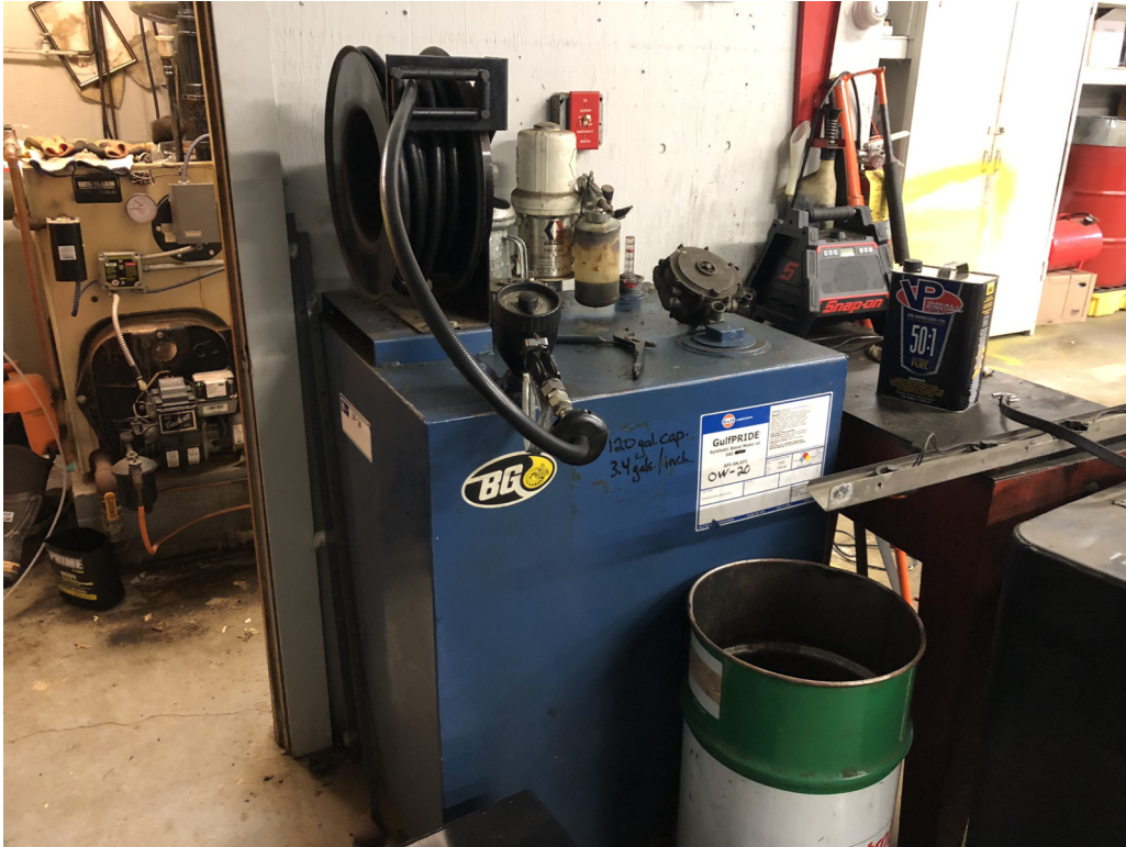
Photo 13: 120-gallon motor oil dispenser on west side of main garage.
