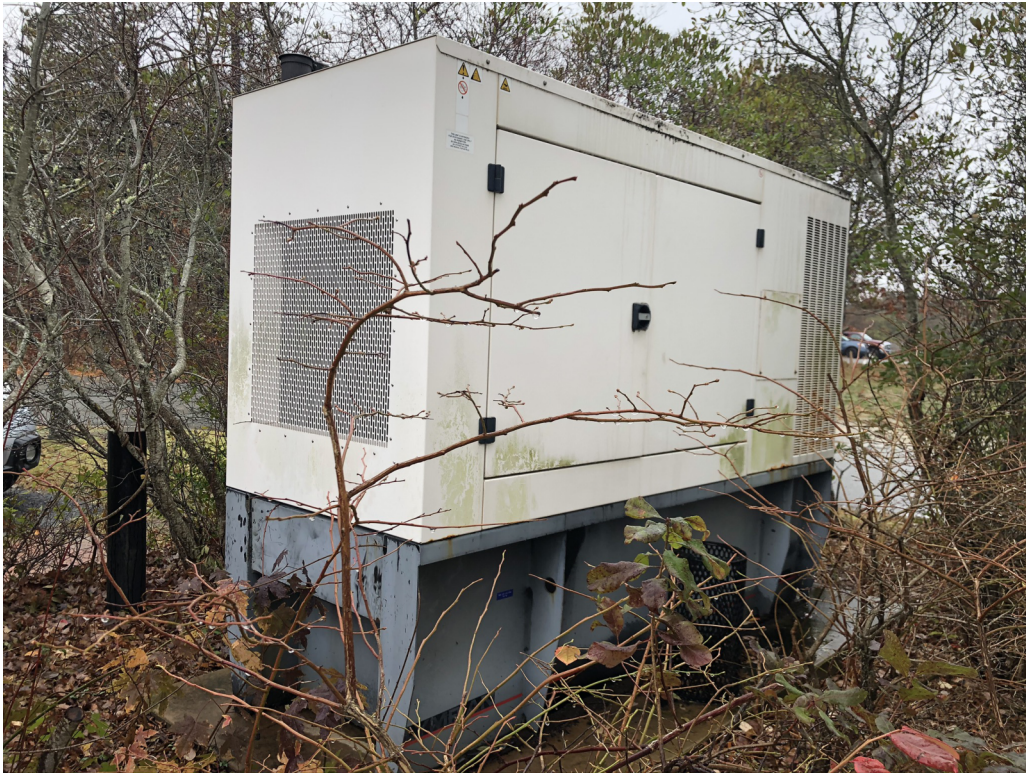
Photo 8: View looking northwest at the Town Hall emergency diesel generator.
