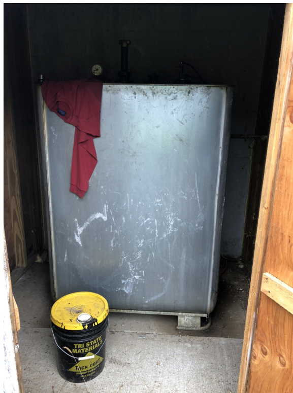
Photo 10: 275-gallon No. 2 fuel oil AST located in detached shed on the west side of the main garage.
