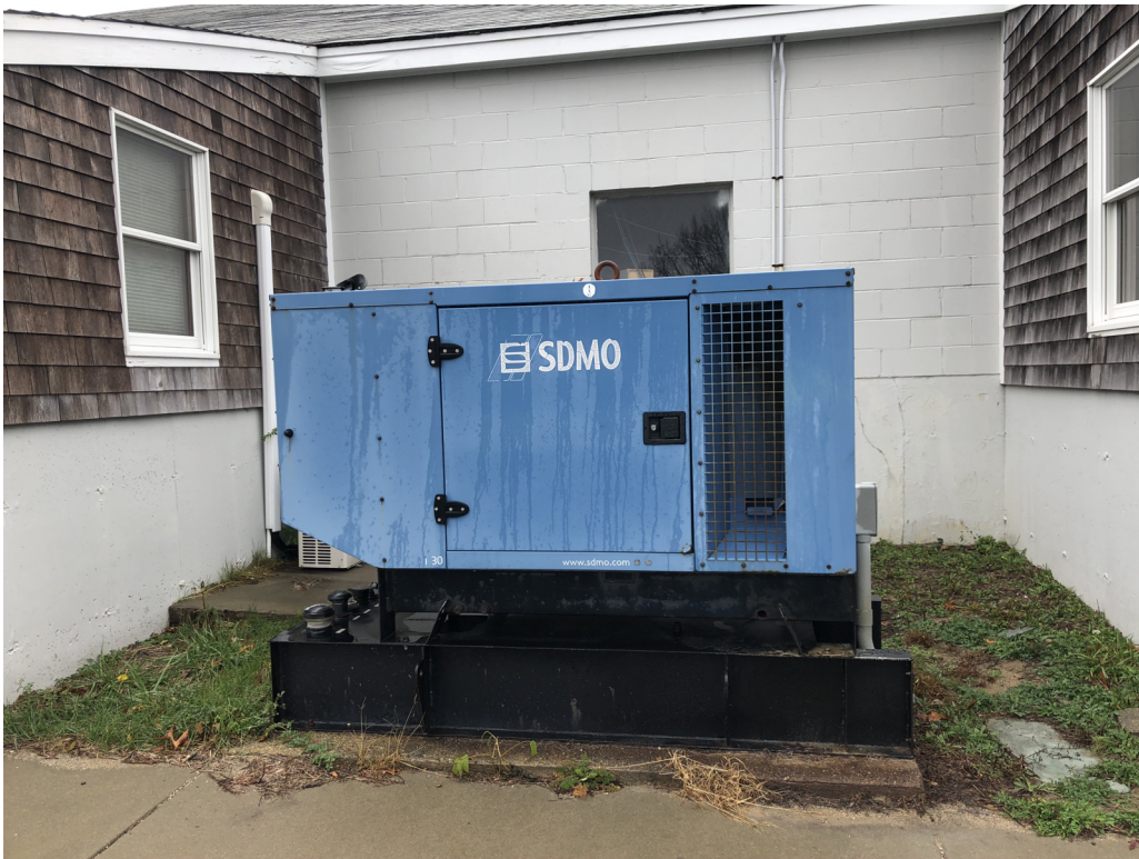
Photo 14: View looking north at the main garage emergency diesel generator.
