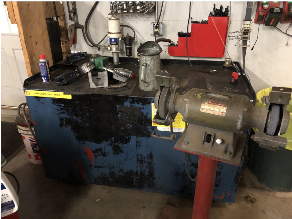
Photo 12: 240-gallon motor oil dispenser on west side of main garage.
