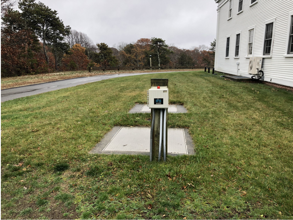
Photo 7: View looking south at the 3,000-gallon underground propane tank.
