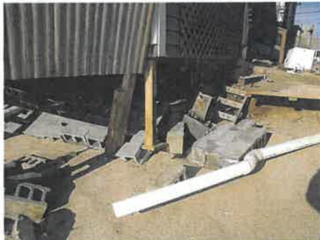
BUILDING 2 FOUNDATION DAMAGE FACING BEACH
