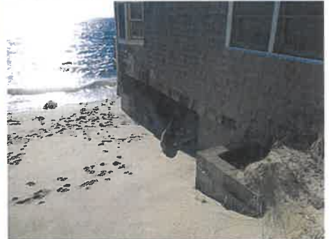
BUILDING 1 FOUNDATION DAMAGE - EAST SIDE
