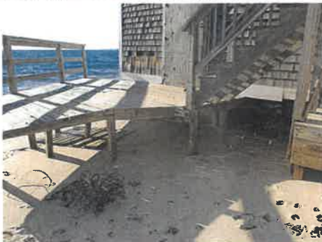
BUILDING 3 REMAINS OF DECK 12-27-2022
