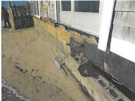
BUILDING 3 FOUNDATION DAMAGE FACING BEACH
