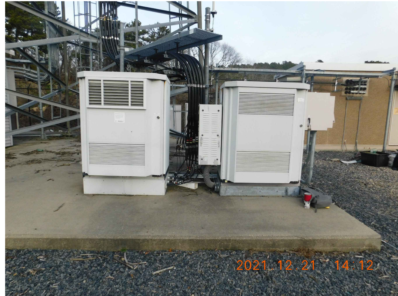
EXISTING EQUIPMENT PHOTO (2/A-1) SCALE: N.T.S.
