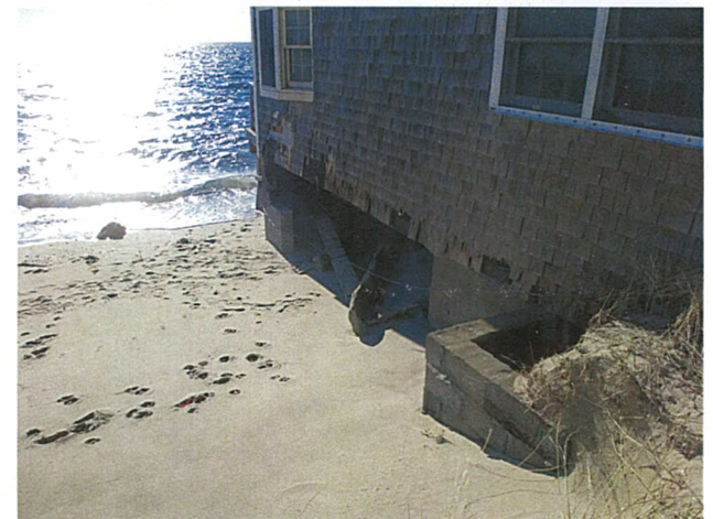
BUILDING 1 FOUNDATION DAMAGE - EAST SIDE
