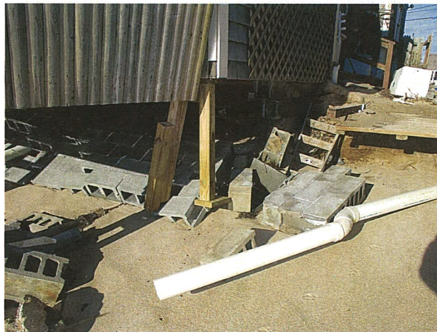
BUILDING 2 FOUNDATION DAMAGE FACING BEACH
