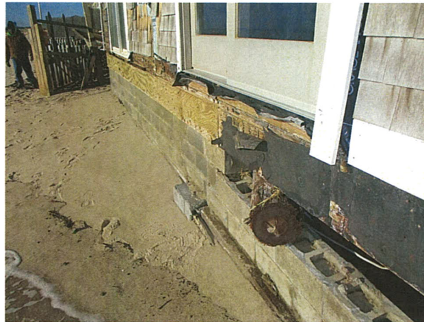
BUILDING 3 FOUNDATION DAMAGE FACING BEACH
