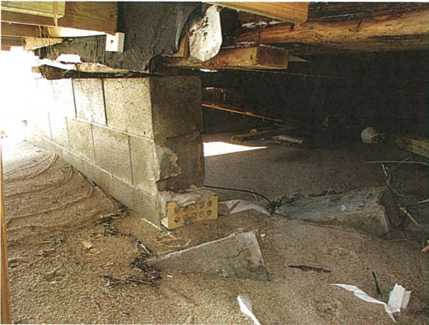
BUILDING 3 FOUNDATION DAMAGE 12-27-22
