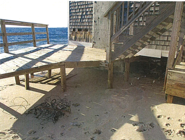
BUILDING 3 REMAINS OF DECK 12-27-2022
