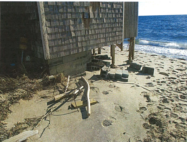
BUILDING 2 FOUNDATION DAMAGE - WEST
