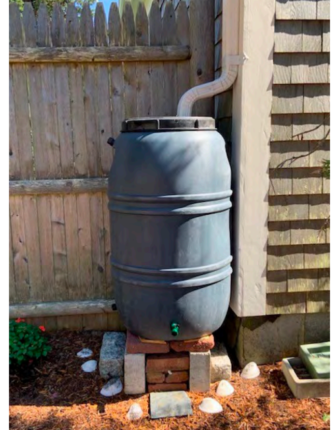
Rain Barrel – Use for Irrigation
