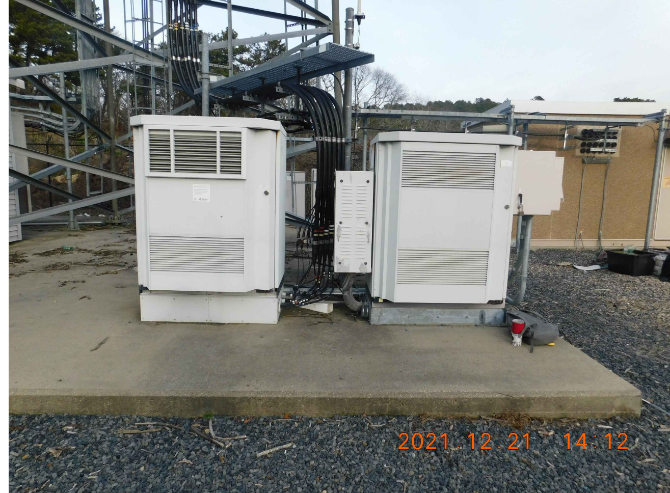
EXISTING EQUIPMENT PHOTO (2/A-1) SCALE: N.T.S.
