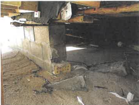
BUILDING 3 FOUNDATION DAMAGE 12-27-22
