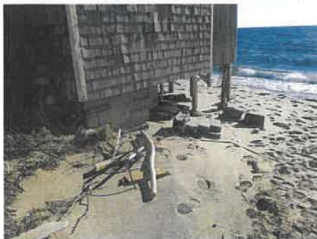
BUILDING 2 FOUNDATION DAMAGE - WEST
