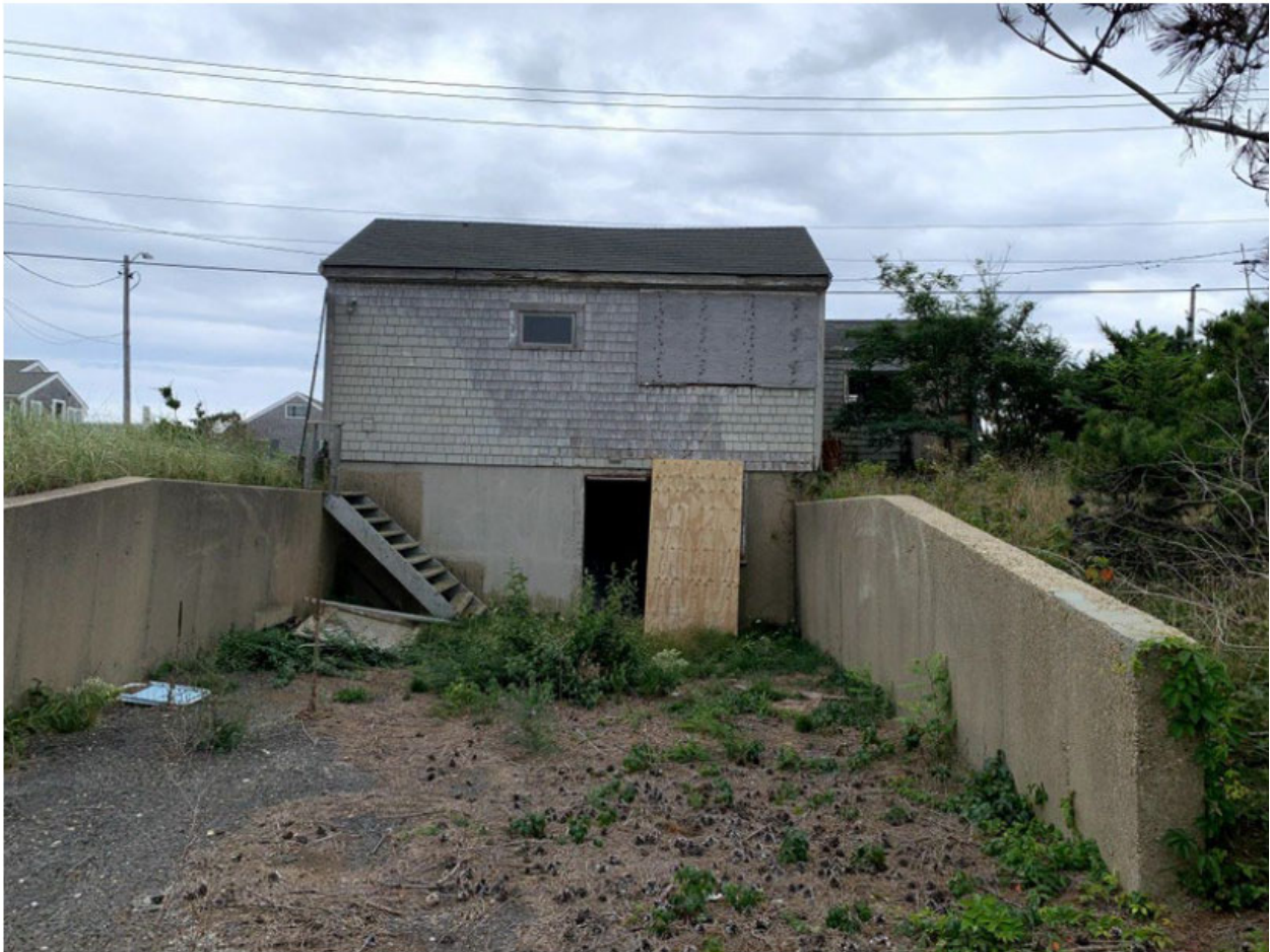
Photo 2: Rear of existing structure at 423 Shore Road (photo by B. Malo, Coastal Engineering Company)
