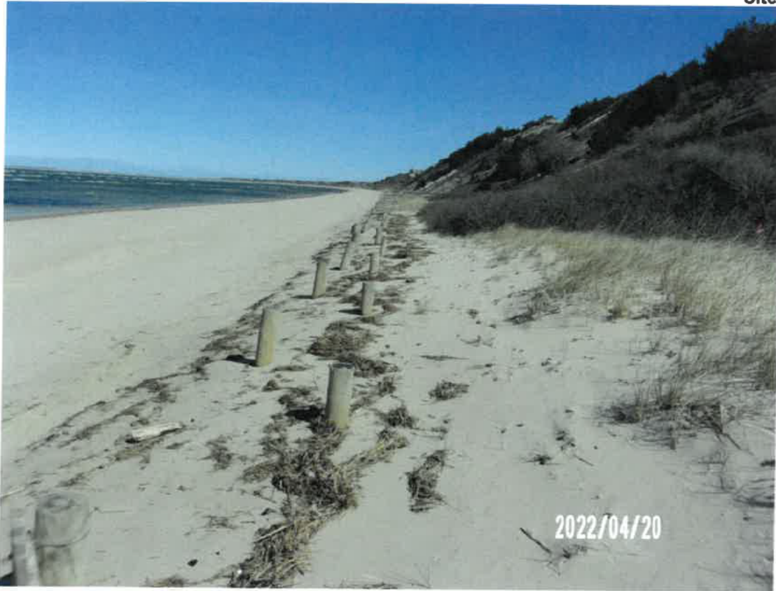
Photograph #3 – Another view north along the existing sand drift fence where much of the fencing sections will need to be replaced.
