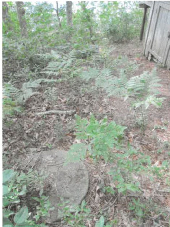
Cover of abandoned septic tank
