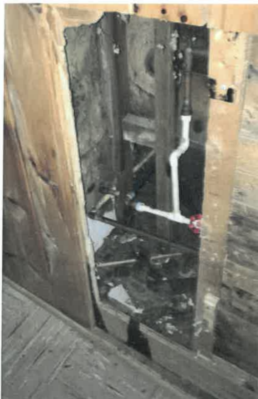
Photo 6 Asbestos Floor Covering & Unfinished Repairs
