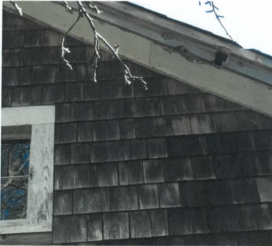
Photo 9 House North Elevation @ Critter Entry Point
