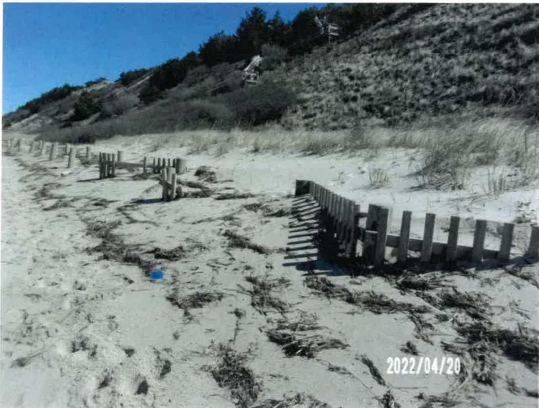
Photograph #2 - View north along the existing sand drift fence. Many existing support piles will need to be raised and resecured.
