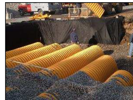
UNDERGROUND INFILTRATION CHAMBERS
