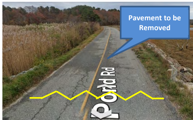
Figure 12 — Approximate Limit of Pavement Removal and Channel Breach South of Mill Pond Culvert (facing south)
