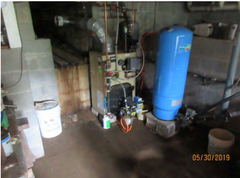
Stained floor in # 7 basement
