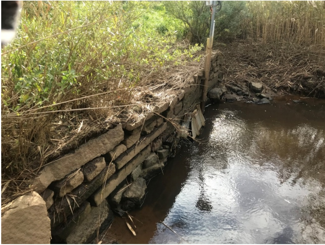
Figure 1. Photo showing the downstream view of Wilder's Dike culvert & flap gate at Truro Center Road over the Pamet River.
