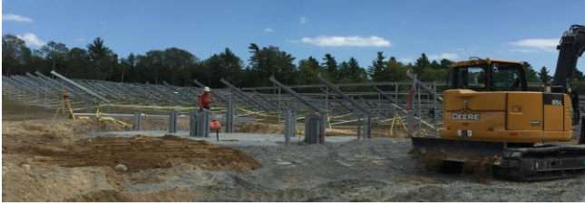
Figure 4. Photo of anchors being installed in preparation for solar racking installation at Dartmouth Farms Solar. Photo courtesy of Nexamp LLC.
