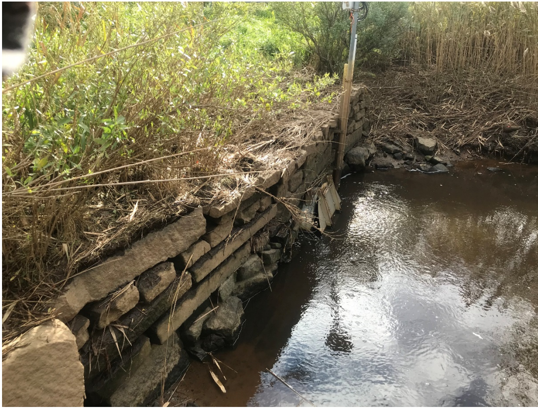
Figure 2. Photo showing the downstream view of Wilder's Dike culvert & flapgate at Truro Center Road over the Pamet River.
