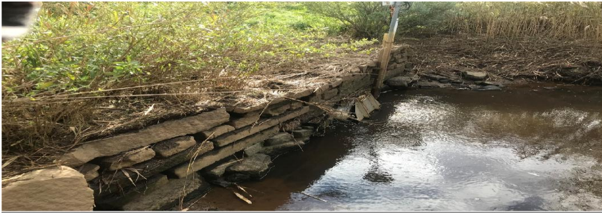
Figure 2. Photo showing the downstream view of Wilder's Dike culvert & flapgate at Truro Center Road over the Pamet River.
