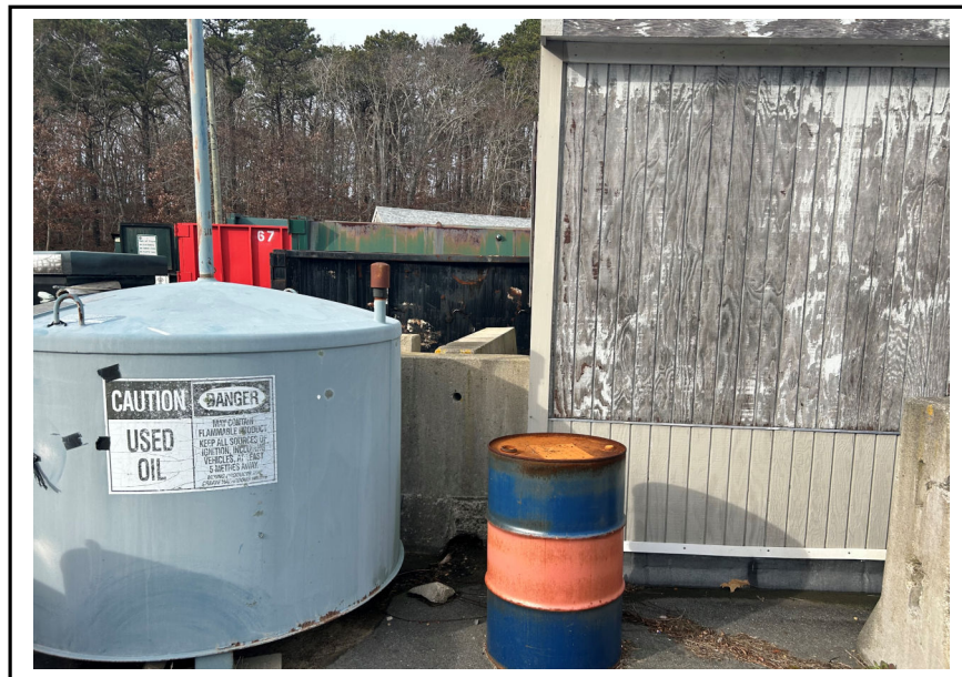
Photo 2: Waste oil AST with a start date noted as November 13, 2023. Accumulation Information is stored in the office. No indication of significant spilling/leaking in the vicinity of the AST.
