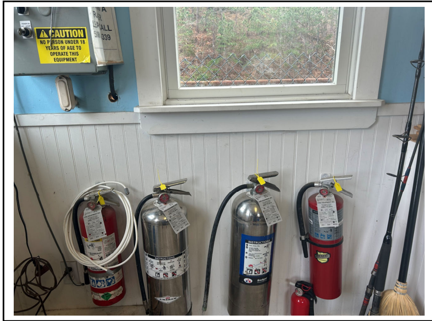
Photo 11: Typical fire extinguisher storage. Extinguishers serviced March 2023 by Fire Equipment Inc. of Hyannis.
