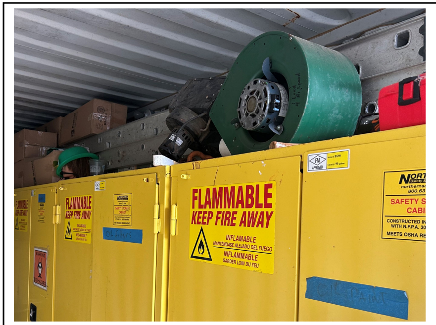
Photo 10: Interior locked flammable storage bins for oil-based paint, sharps and other hazardous materials.
