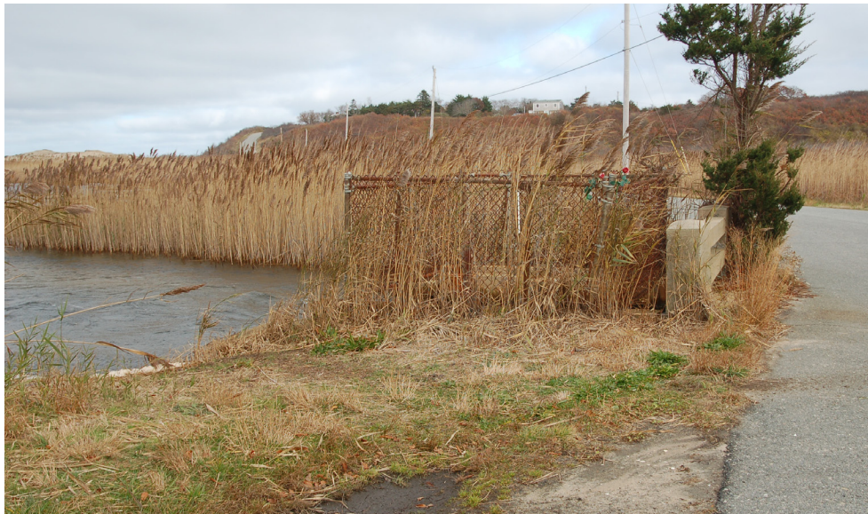
Figure 2.2b | High Head Road Culvert owned by the National Park Service. Built in 1956. These photographs were taken during an extreme high tide. Note that the water level is close to the road level.
