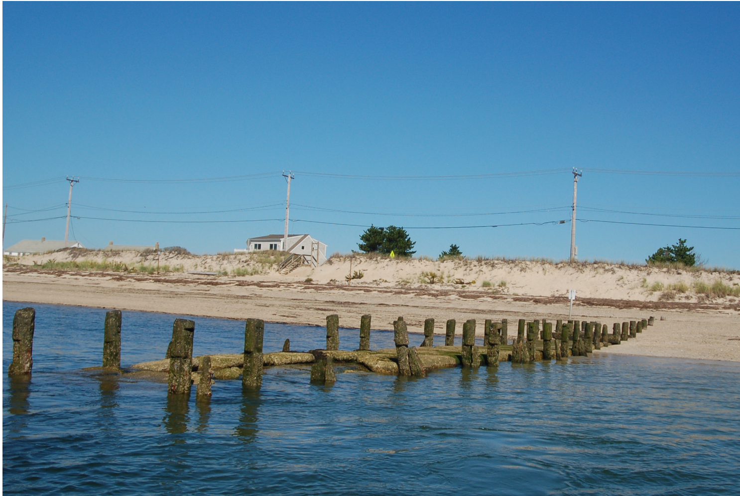
Figure 2.2c | The outfall pipe of the East Harbor culvert, owned by the Town of Truro..
