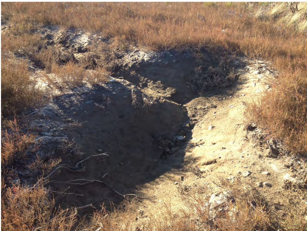
Figure 2-5. Slumping of cover fill over the East Harbor culvert between Shore Road and Route 6.
