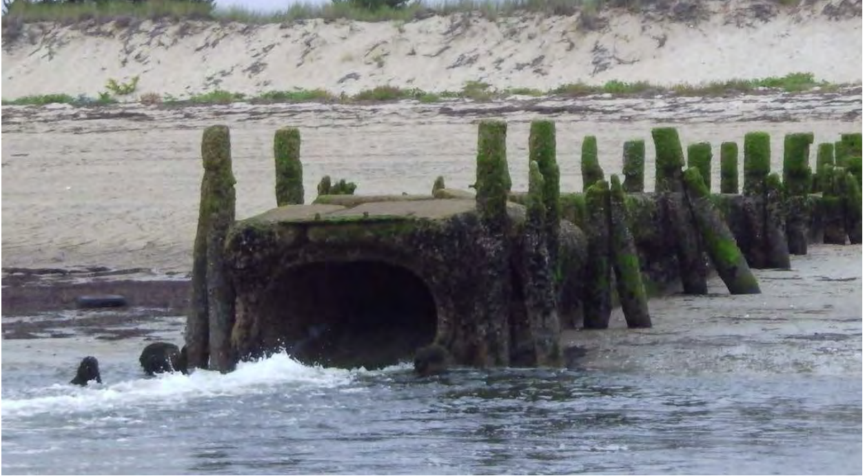
Figure 2-3b. Water side view of the failing portion of the East Harbor culvert in Cape Cod Bay. Pitched/misaligned seaward section noted also with no debris rack.
