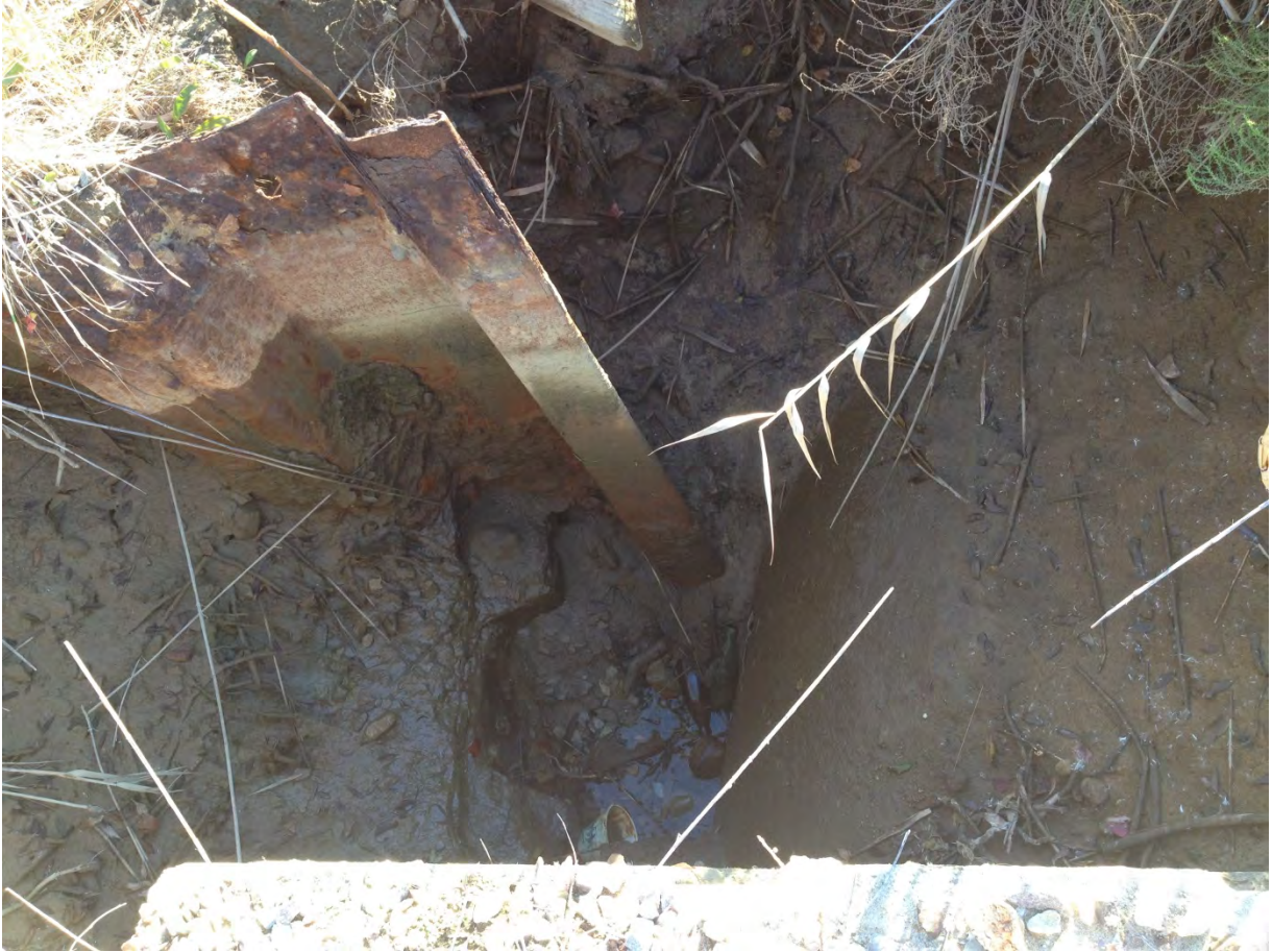
Figure 2-6. Slumping of cover fill material near the junction box connected to Route 6.
