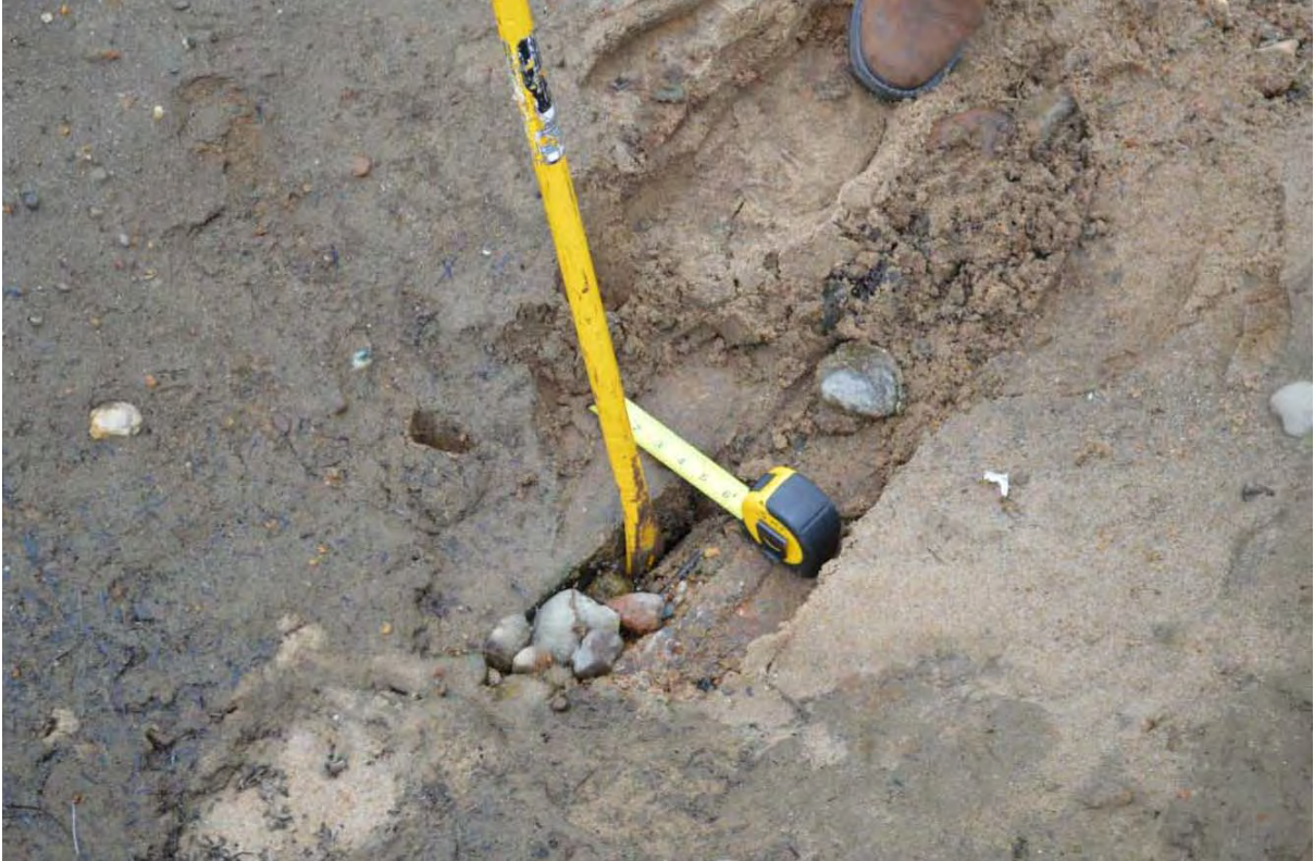
Figure 2-7. Failing joint between culvert sections.
