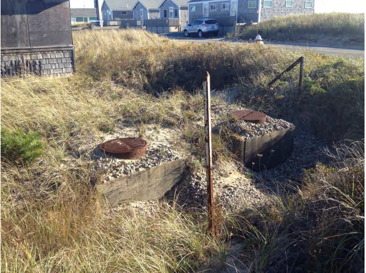
Figure 2-4. Slumping of cover fill near the junction box landward of Shore Road.
