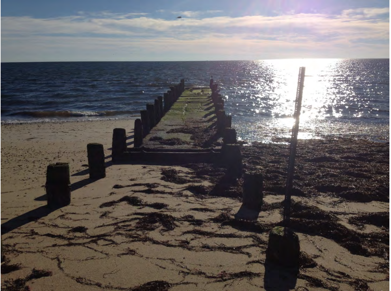
Figure 2-3a. Seaward portion of East Harbor culvert. Terminus sections are failing, including slumping into the Bay as well as removal of the protective safety and debris grate.
