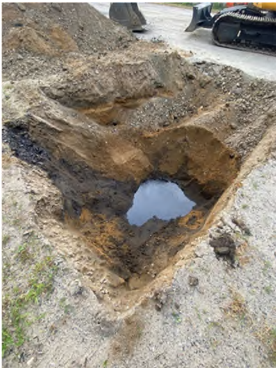
Photo 3: View of petroleum in TP-5 beneath tank and drums
